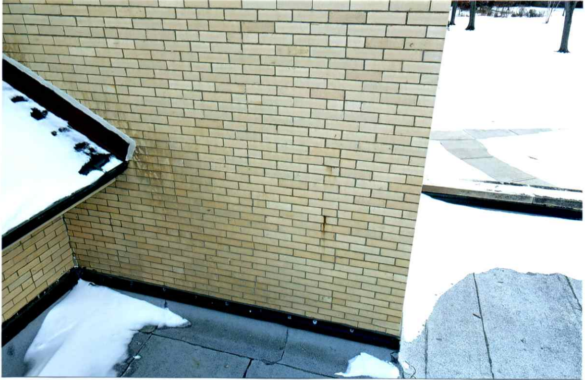
Photo 73. Good condition of the square region above the building roof (north side).
