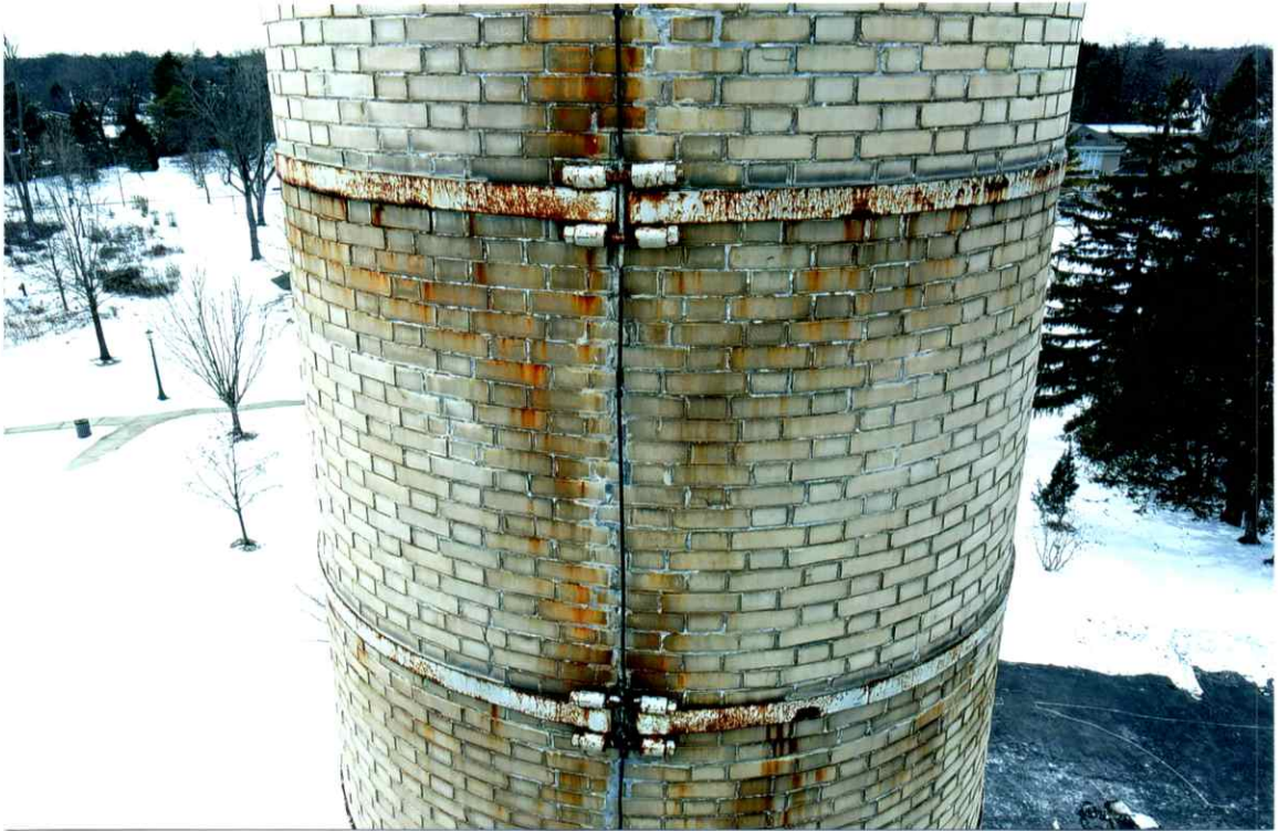
Photo 43. Good exterior condition of the east side local to the 61' level. Mortar joints were only slightly weathered. Repairs to the crack were sound (see Photo 49).
