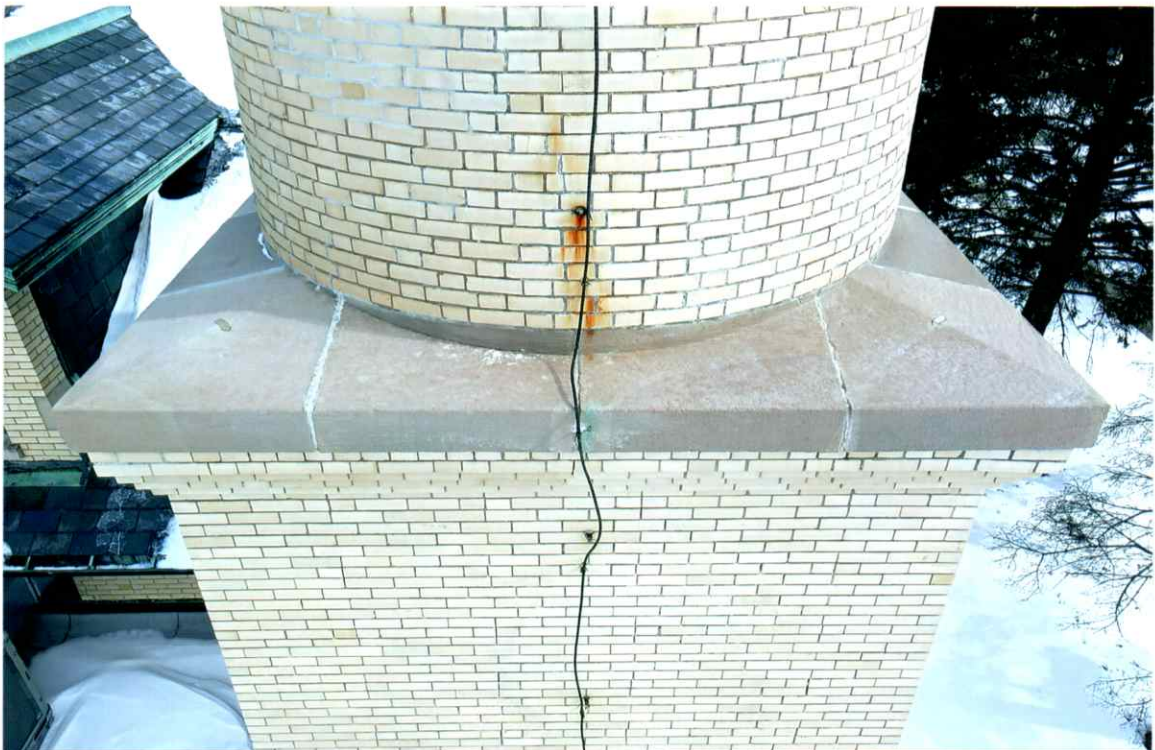
Photo 72. Good condition of the stone transition and corbelled square regions (29' level, west side). A few open and recessed mortar joints were observed.
