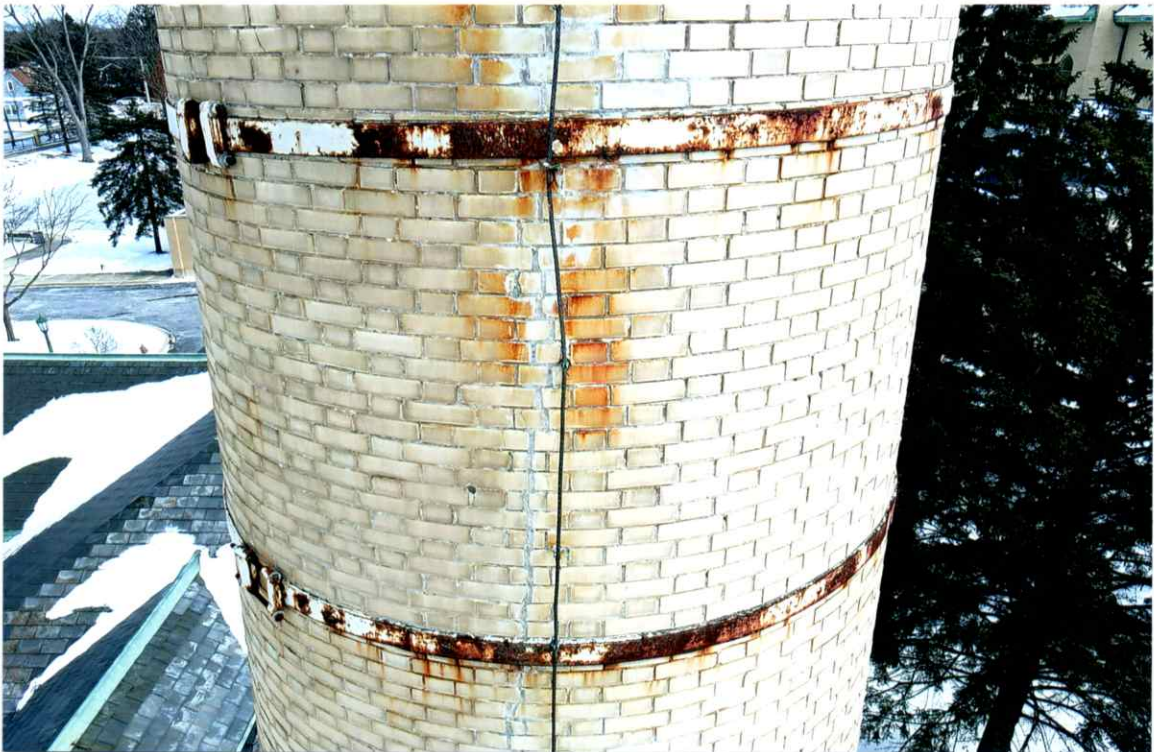
Photo 54. Good exterior condition of the west side local to the 50' level. Mortar joints were only slightly weathered. Repairs to the crack were sound.
