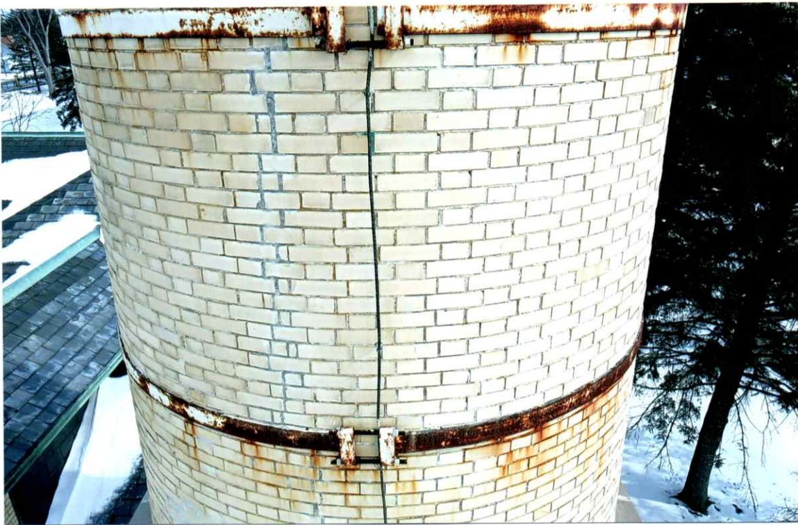
Photo 64. Good exterior condition of the west side local to the 38' level. Mortar joints were only slightly weathered. Note the rust on the bands.
