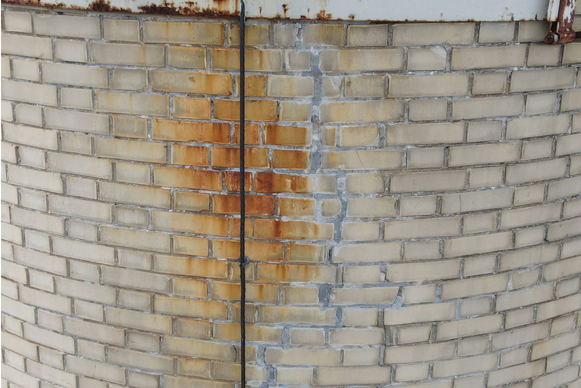
Photo 59. Close-up of the good condition of the repaired crack (east side, 50' level).
