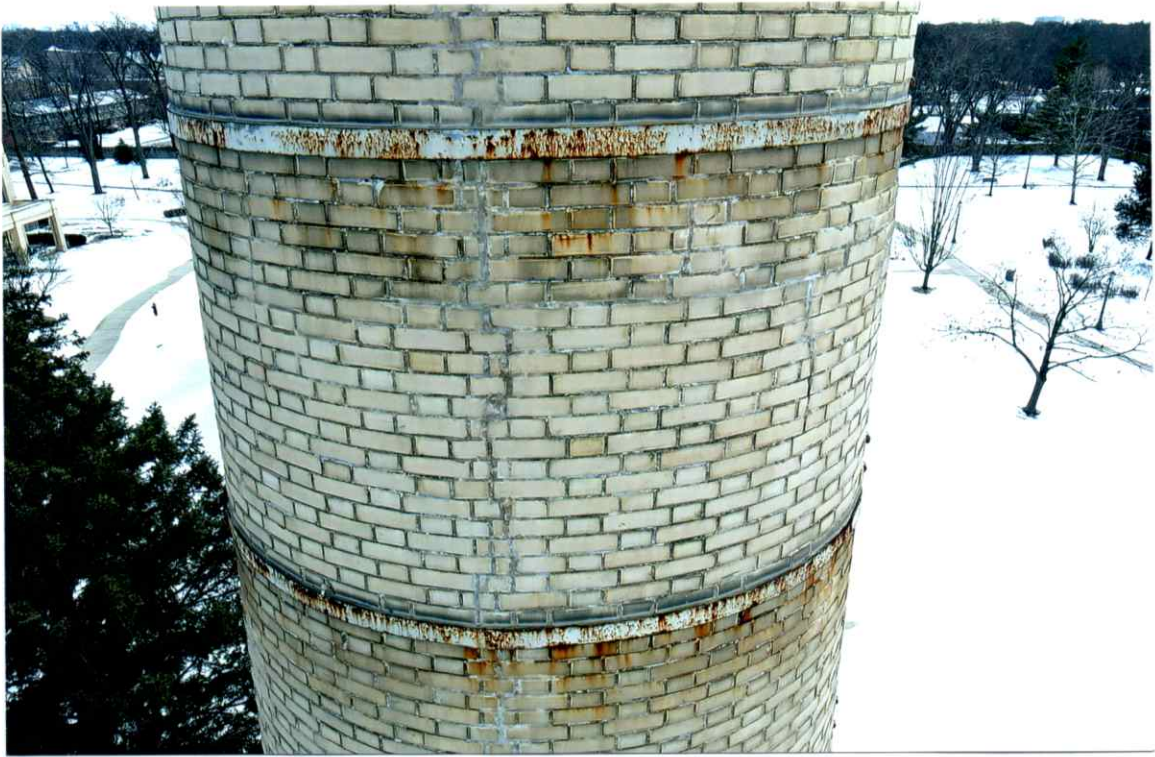
Photo 35. Fair exterior condition of the north side local to the 67' level. Mortar joints were weathered and recessed. Repairs to the crack were in fair condition (see Photo 40).
