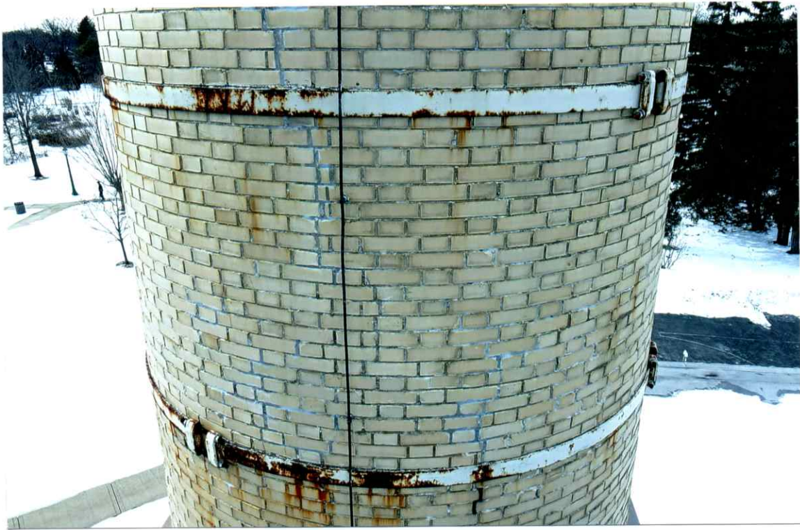
Photo 63. Good exterior condition of the east side local to the 38' level. Mortar joints were only slightly weathered. Note the rust on the bands.
