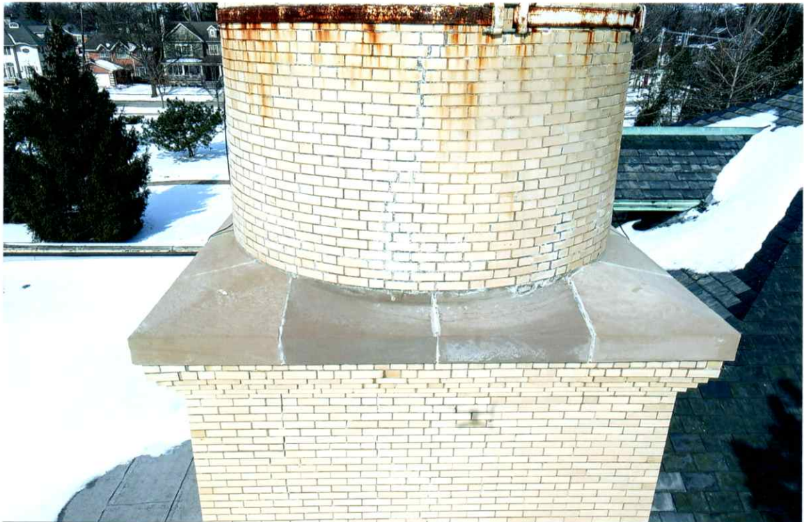
Photo 66. Good exterior condition of the south side local to the 32' level. Mortar joints were only slightly weathered. Repairs to the crack were sound.
