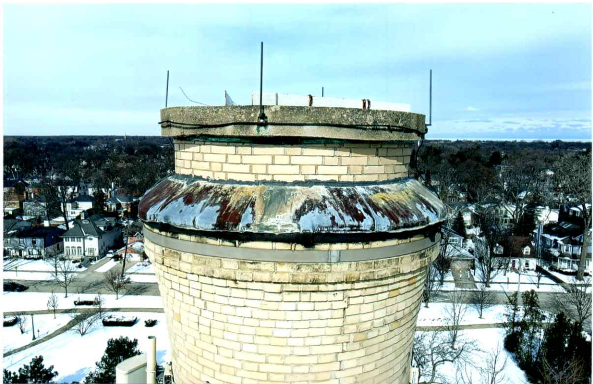
Photo 8. Overall good condition of the upper elevations of the south side. The uppermost exterior band and flashing were secure. A few open mortar joints were noted.
