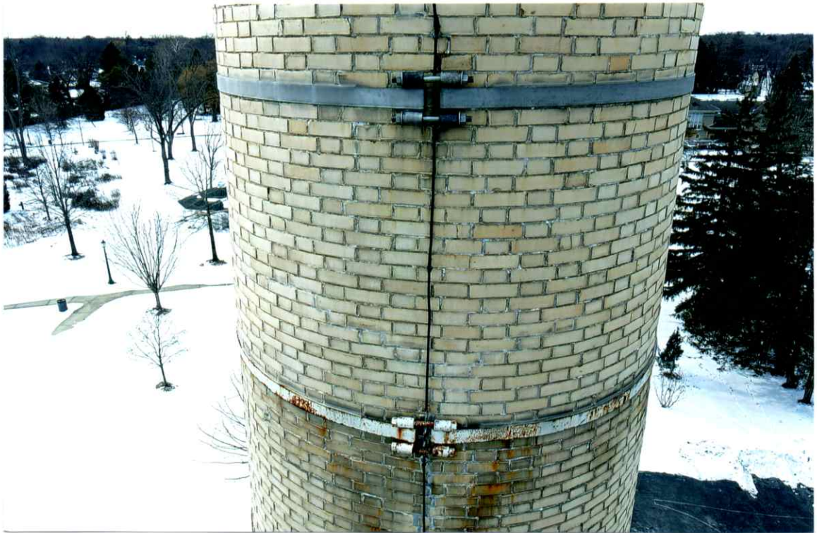
Photo 33. Fair exterior condition of the east side local to the 73' level. All bands were secure. Mortar joints were weathered and recessed.
