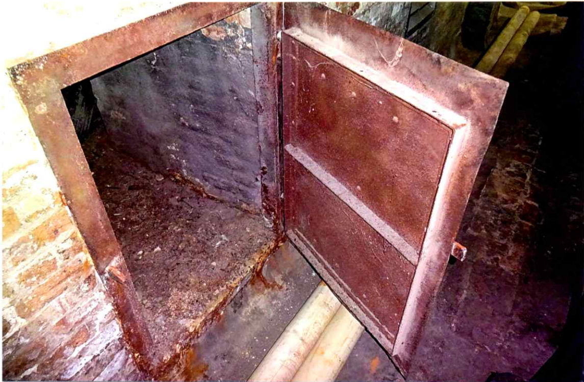
Photo 80. Fair interior condition of the cleanout door at the base of the east wall.
