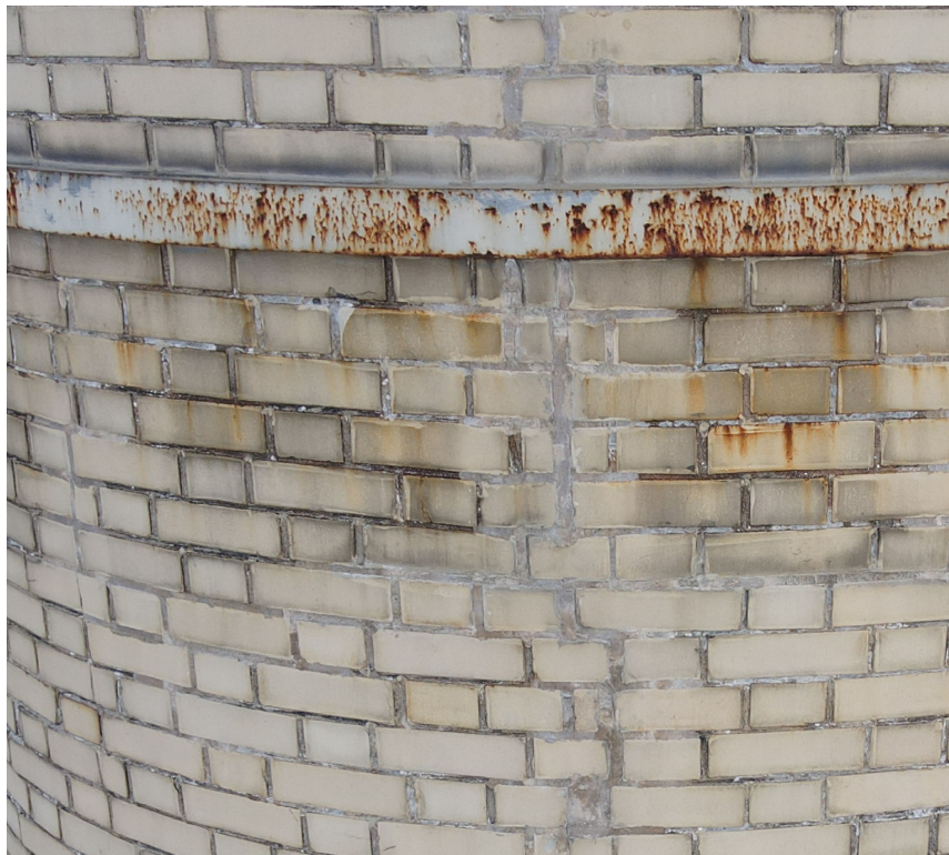
Photo 40. Close-up of the good condition of the repaired crack (north side, 67' level).
