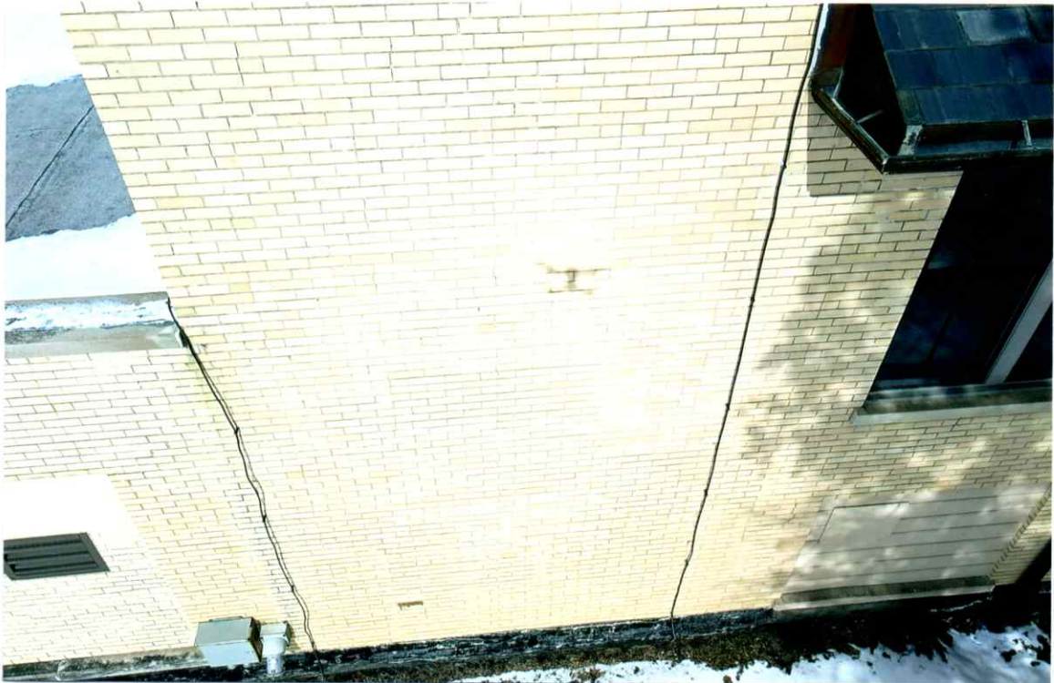
Photo 74. Good condition of the square region in the 25' region above grade (south side). Both LPS downlead cables were properly grounded at grade.
