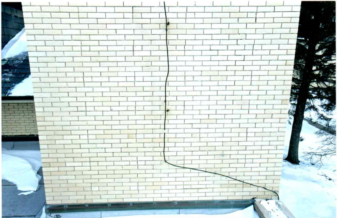
Photo 76. Good condition of the square region above the building roof (west side).
