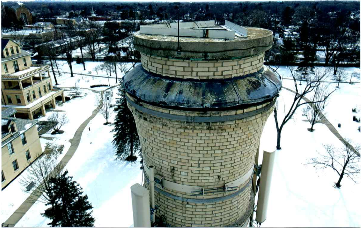
Photo 7. Overall good condition of the upper elevations of the north side. The uppermost exterior band and flashing were secure. Mortar joints were slightly weathered.
