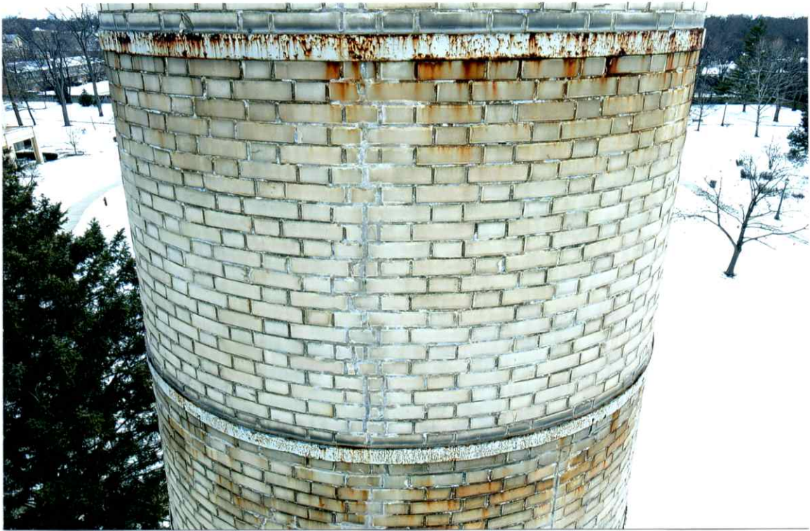
Photo 41. Good exterior condition of the north side local to the 61' level. Mortar joints were only slightly weathered. Repairs to the crack were sound.
