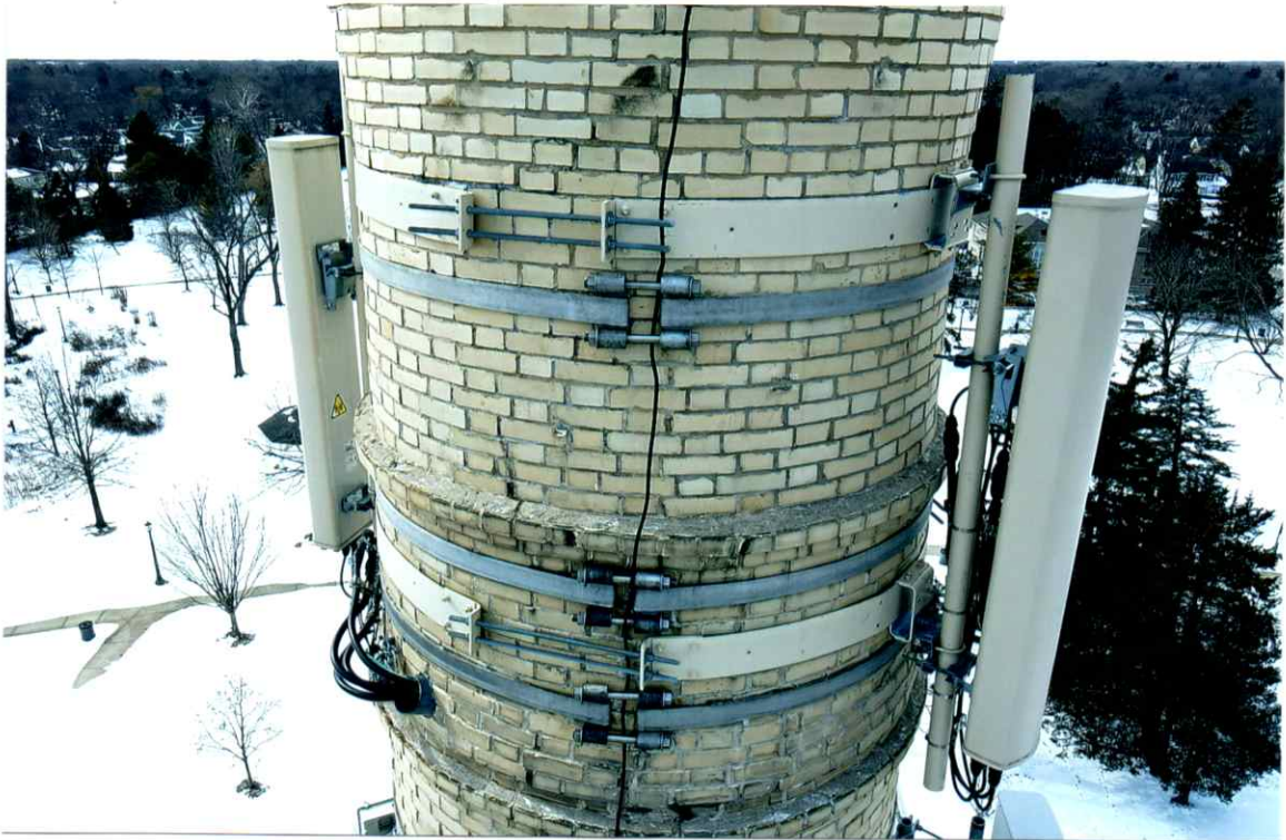
Photo 13. Overall good condition of the east side local to the upper level of antenna. All antennas and antenna support components were secure. Mortar joints were slightly weathered.
