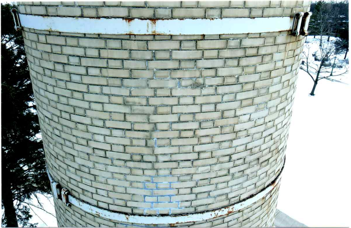
Photo 55. Good exterior condition of the north side local to the 44' level. Mortar joints were only slightly weathered. Repairs to the crack were sound.
