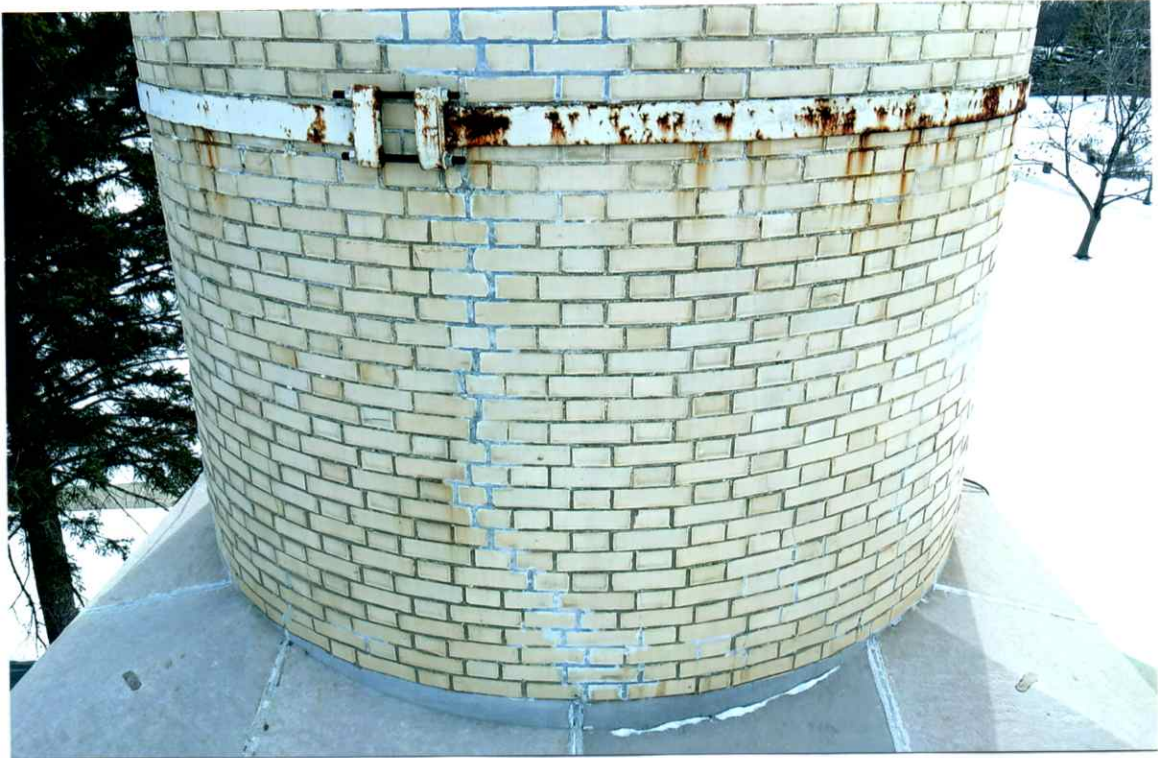
Photo 65. Good exterior condition of the north side local to the 32' level. Mortar joints were only slightly weathered. Repairs to the crack were sound.
