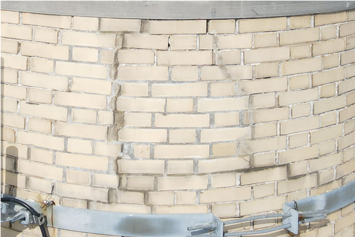
Photo 19. Close-up of the good condition of the repaired crack (south side, 93' level).
