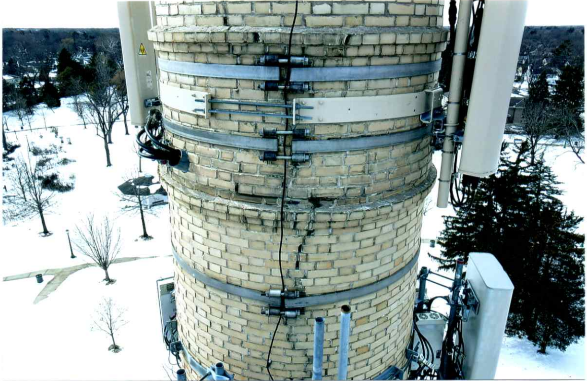
Photo 17. Fair exterior condition of mortar joints near the 93' level (east side). Past repairs to the crack were in poor condition (see Photo 20).
