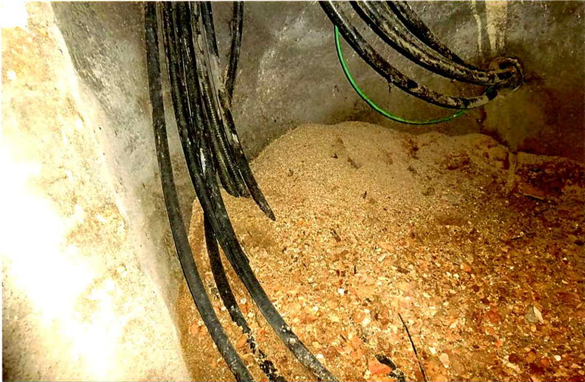
Photo 83. 8" of accumulated debris in the base (south side).
