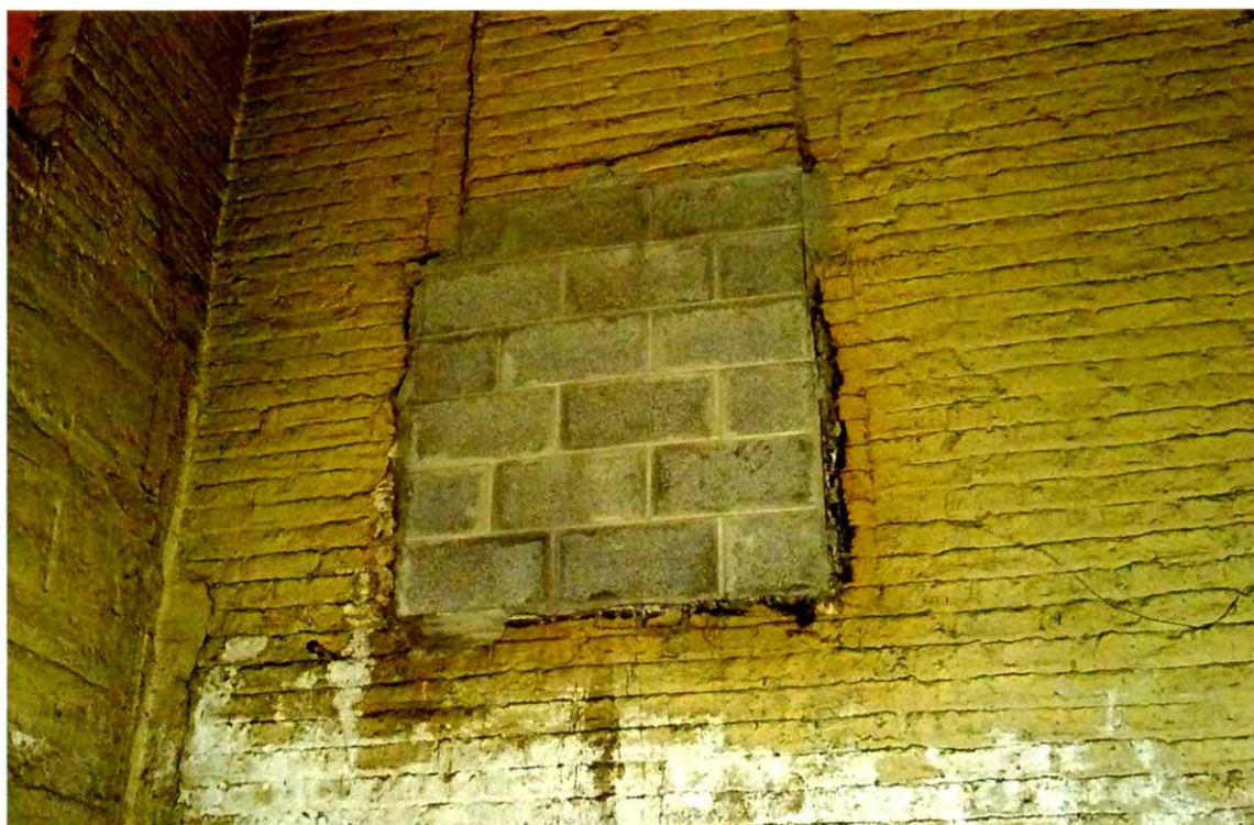
Photo 78. Close-up of the blocked up boiler duct opening (east side, sill near grade).
