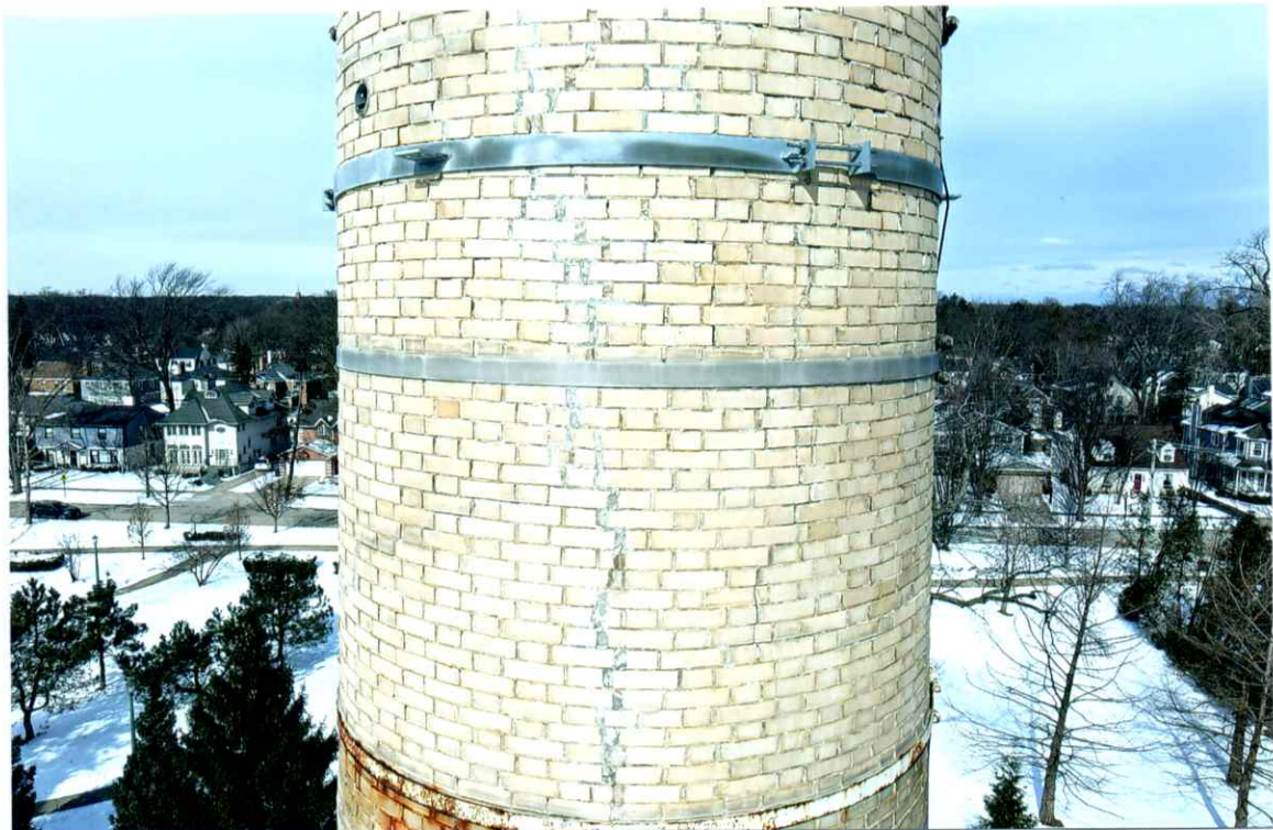
Photo 32. Fair exterior condition of the south side local to the 73' level. All bands were secure. Past repairs along the crack were sound.
