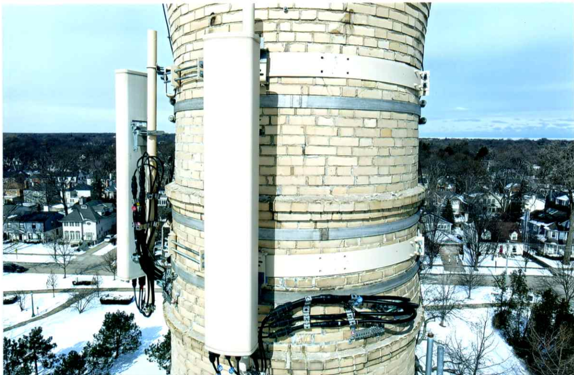
Photo 12. Overall good condition of the south side local to the upper level of antenna. All antennas and antenna support components were secure. Mortar joints were slightly weathered.
