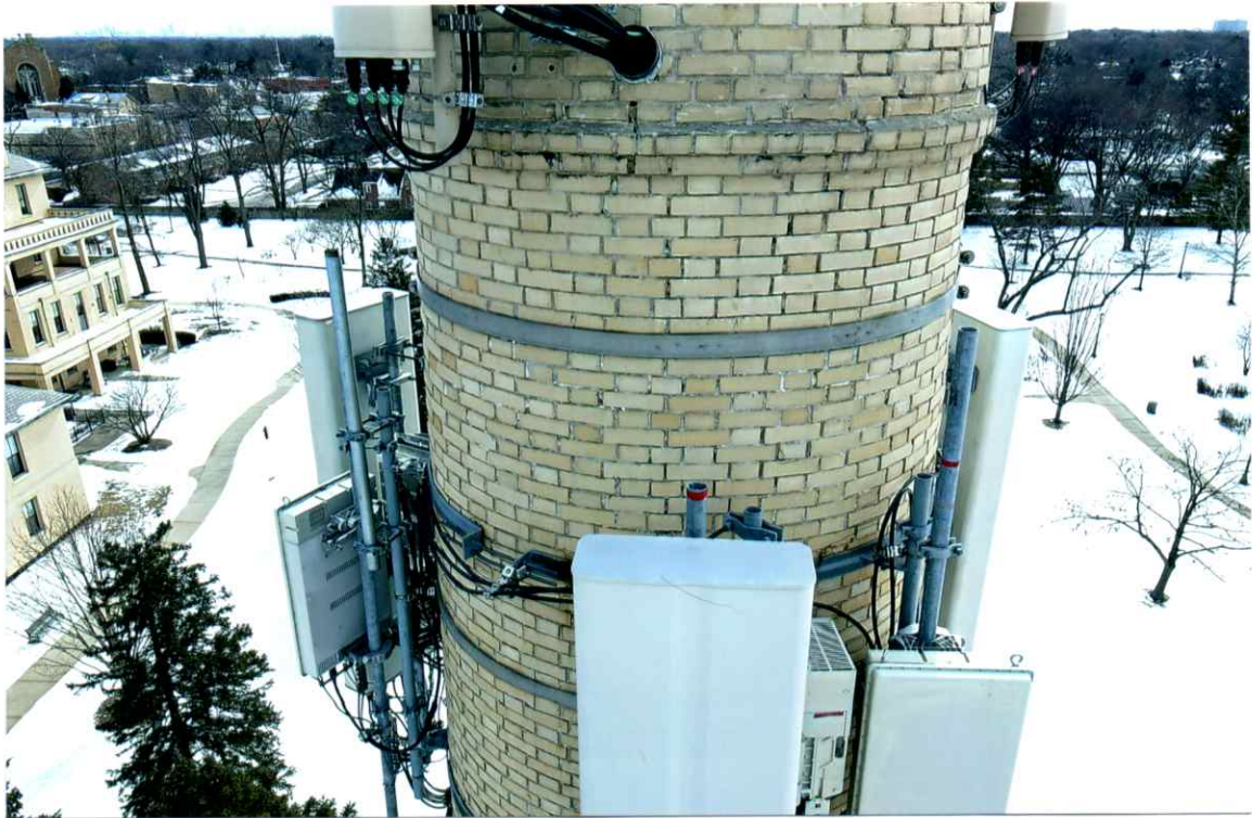
Photo 15. Fair exterior condition of mortar joints near the 93' level (north side). Mortar joints were slightly eroded and recessed in this region.
