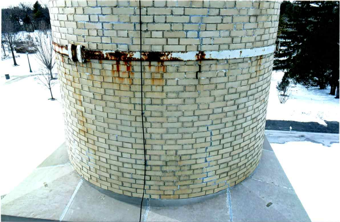
Photo 67. Good exterior condition of the east side local to the 32' level. Mortar joints were only slightly weathered. Repairs to the cracks were sound.
