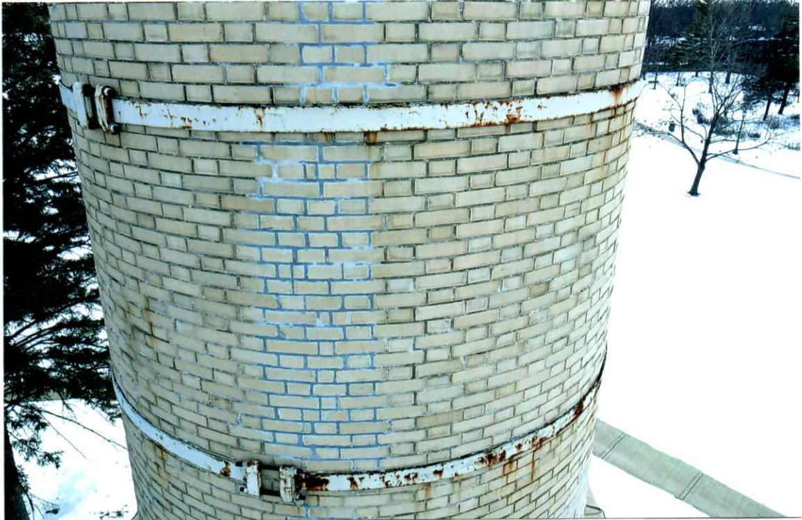
Photo 61. Good exterior condition of the north side local to the 38' level. Mortar joints were only slightly weathered. Note the rust on the bands.
