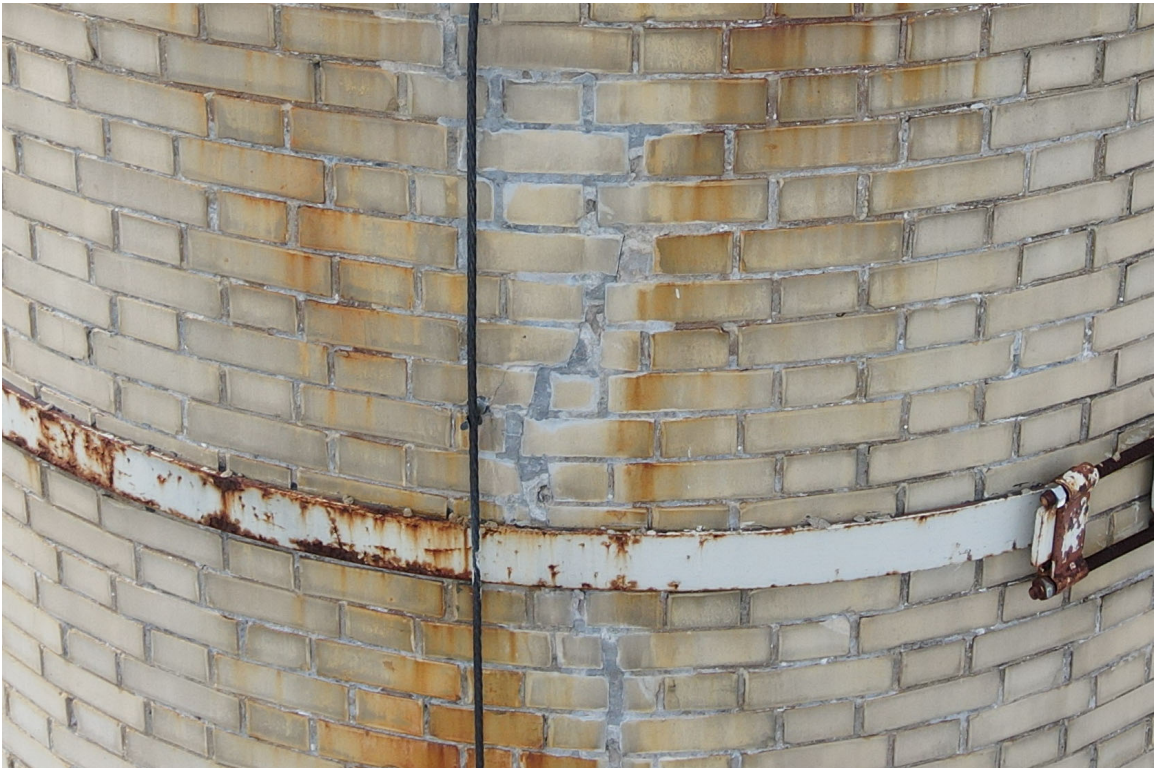
Photo 50. Close-up of the good condition of the repaired crack (east side, 56' level).
