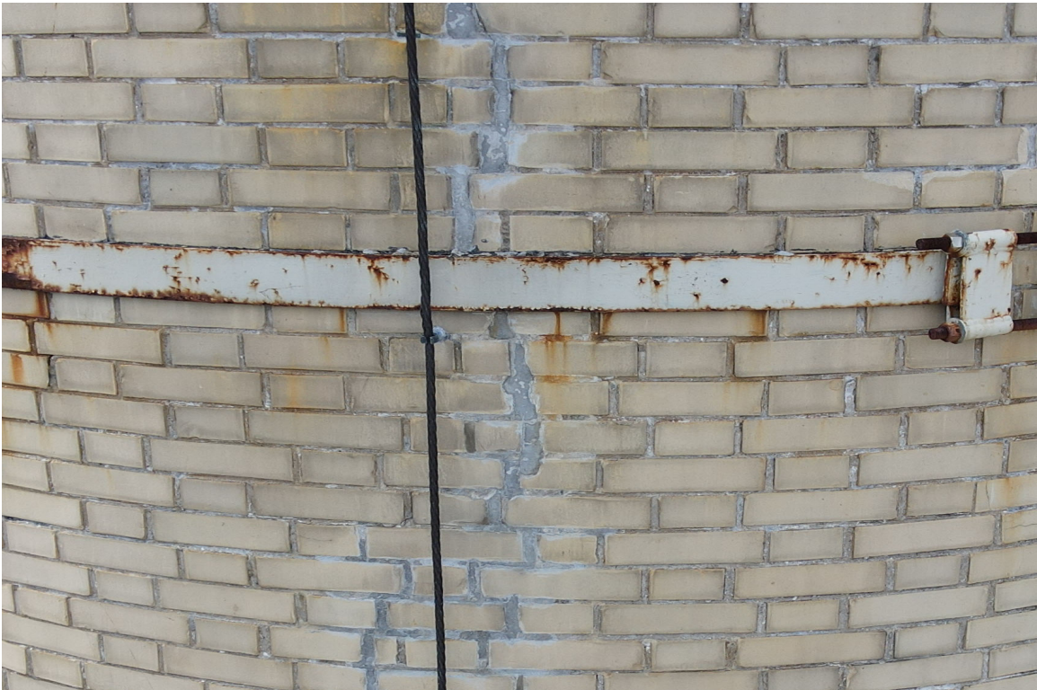
Photo 60. Close-up of the good condition of the repaired crack (east side, 44' level).
