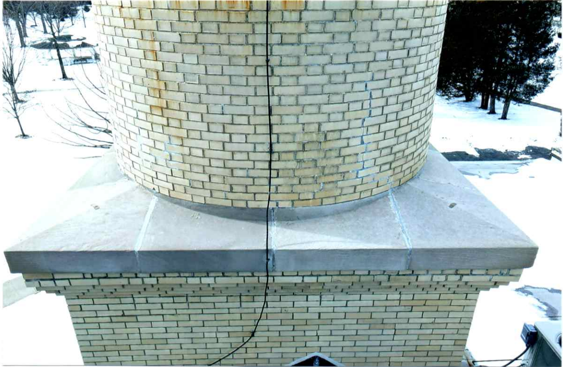
Photo 71. Good condition of the stone transition and corbelled square regions (29' level, east side). A few open and recessed mortar joints were observed.
