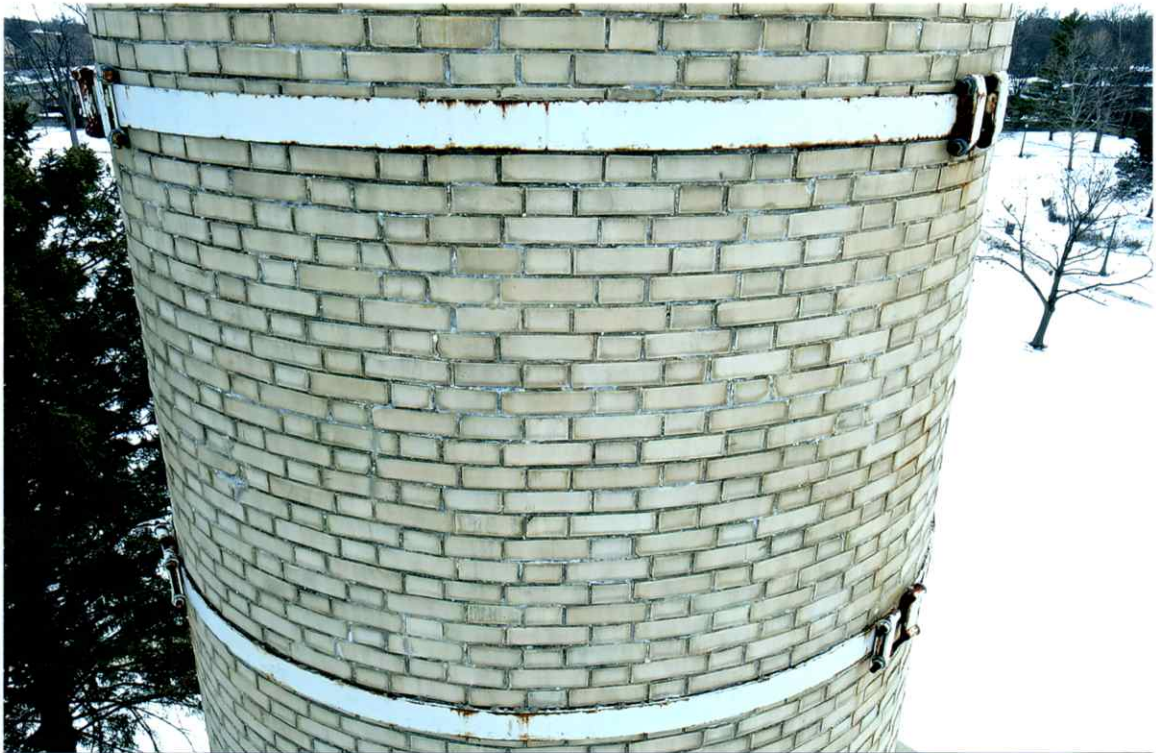
Photo 51. Good exterior condition of the north side local to the 50' level. Mortar joints were only slightly weathered. All bands were secure.
