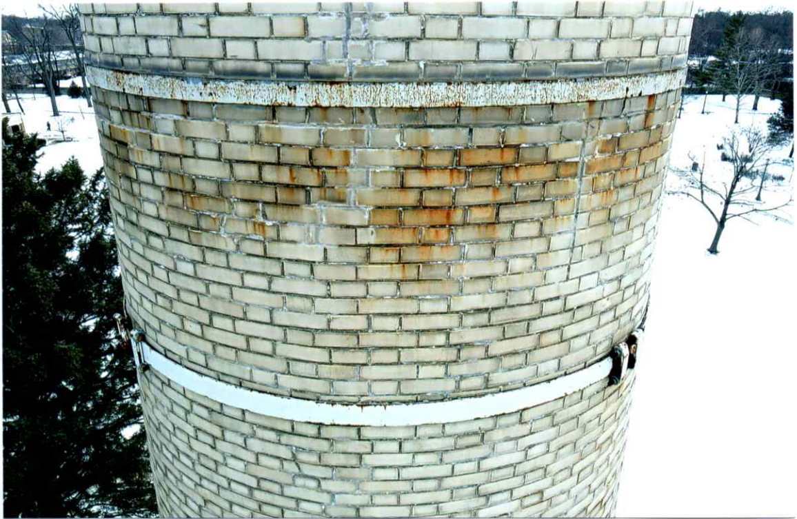
Photo 45. Good exterior condition of the north side local to the 56' level. Mortar joints were only slightly weathered. Repairs to the crack were sound.
