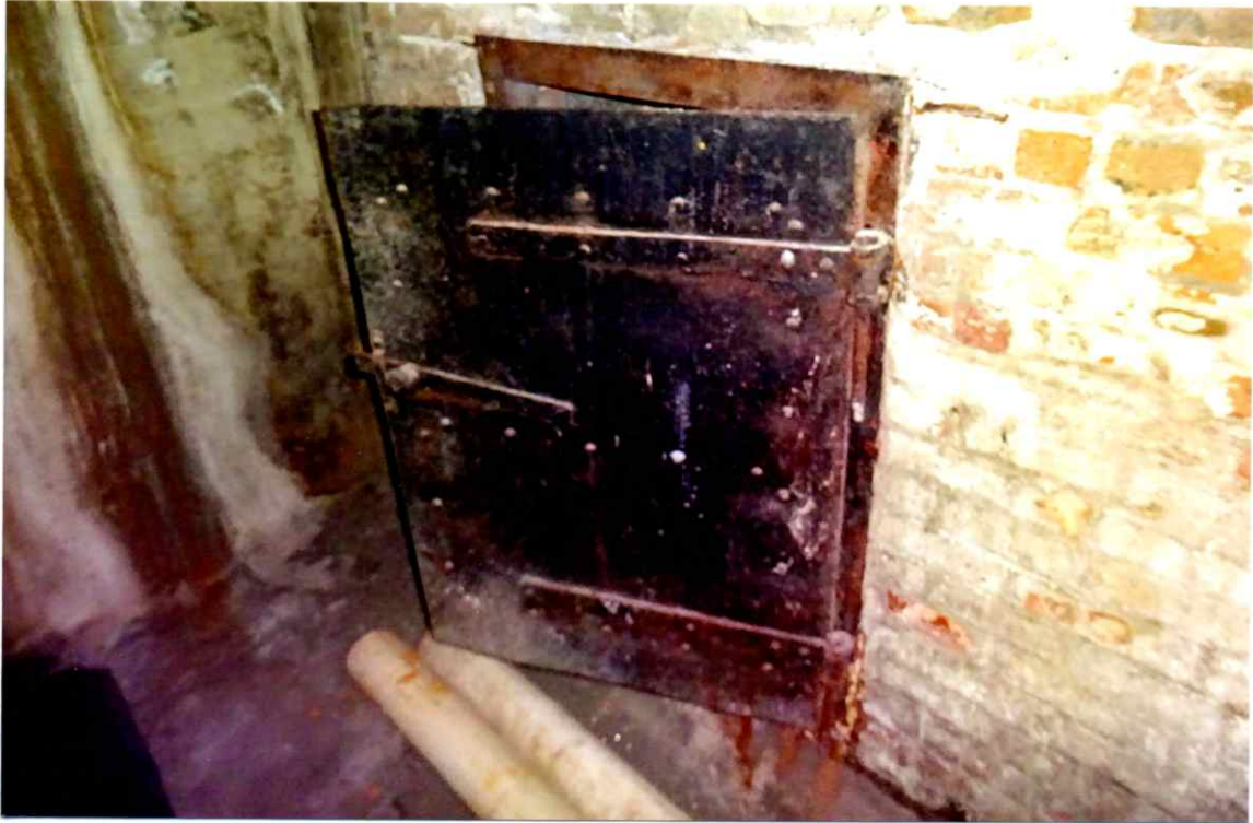
Photo 79. Good exterior condition of the cleanout door at the base of the east wall.
