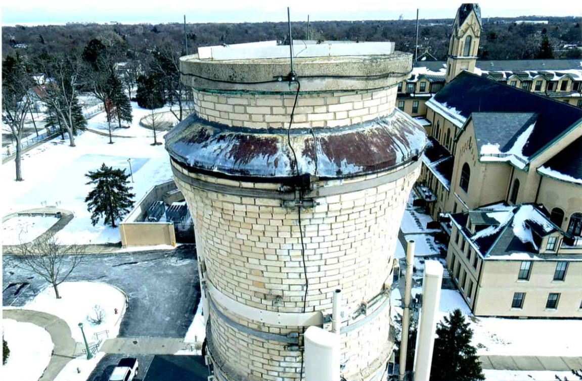
Photo 10. Overall good condition of the upper elevations of the west side. The uppermost exterior band and flashing were secure. Mortar joints were slightly weathered.
