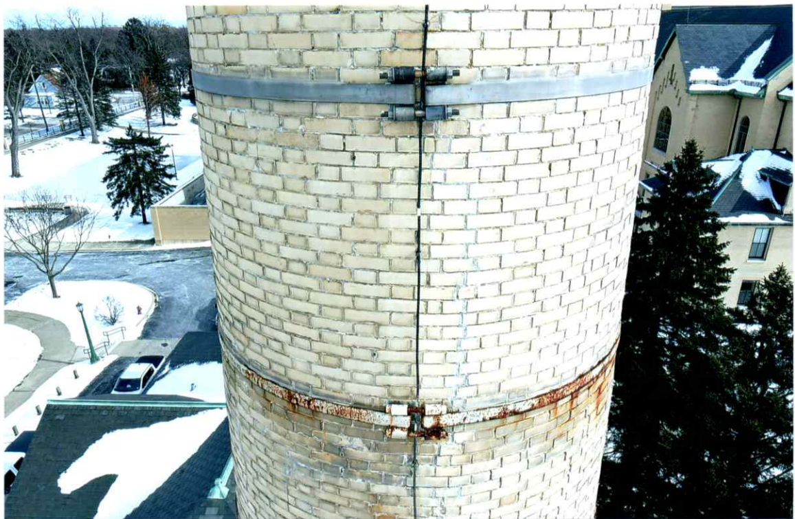
Photo 34. Fair exterior condition of the west side local to the 73' level. All bands were secure. Mortar joints were weathered and recessed.
