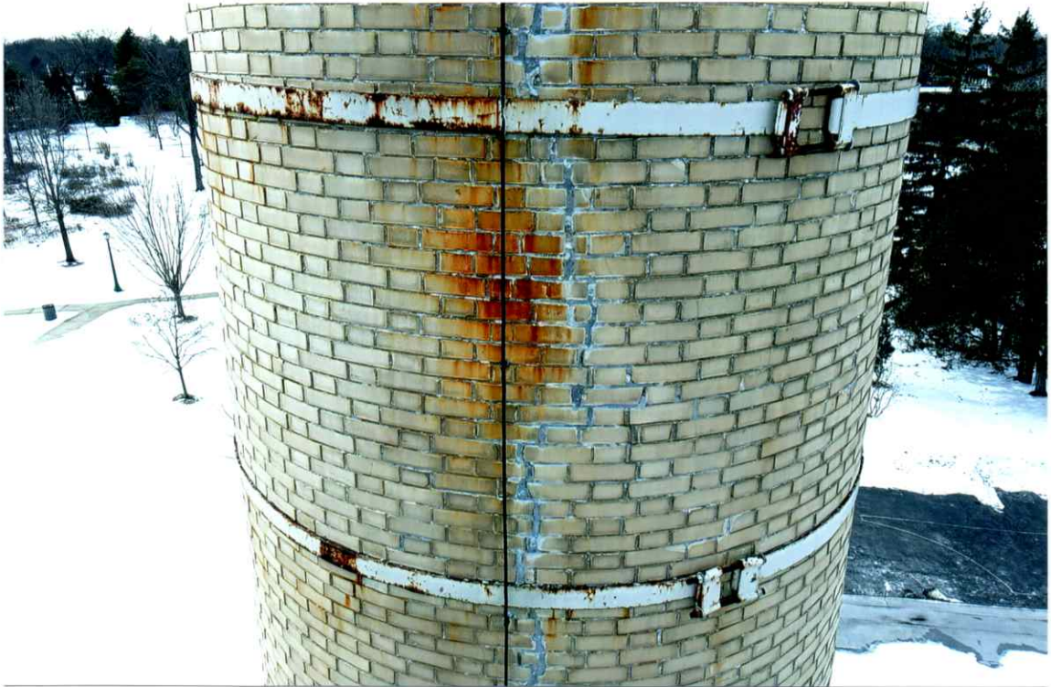
Photo 53. Good exterior condition of the east side local to the 50' level. Mortar joints were only slightly weathered. Repairs to the crack were sound (see Photo 59).
