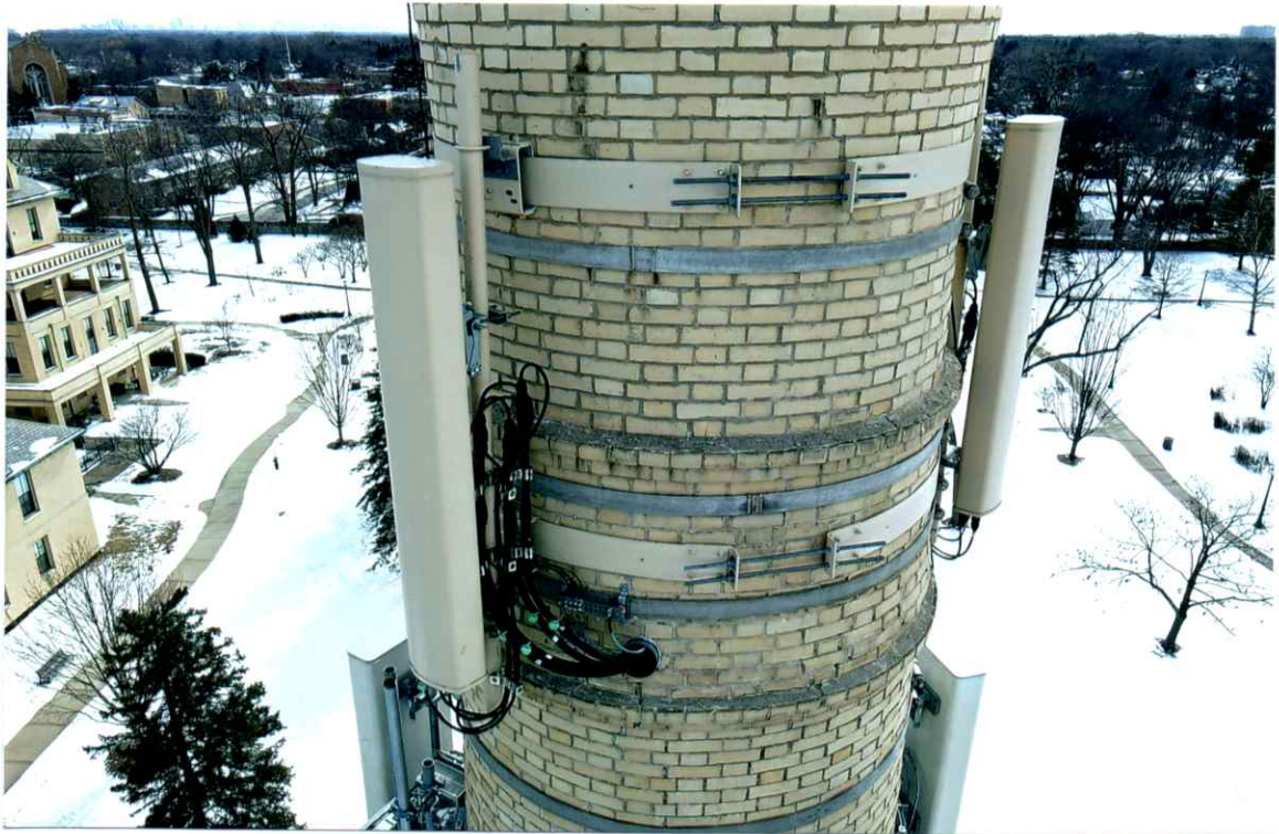
Photo 11. Overall good condition of the north side local to the upper level of antenna. All antennas and antenna support components were secure. Mortar joints were slightly weathered.
