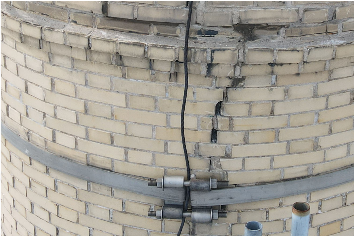
Photo 20. Close-up of the poor condition of the repaired crack (south side, 93' level).
