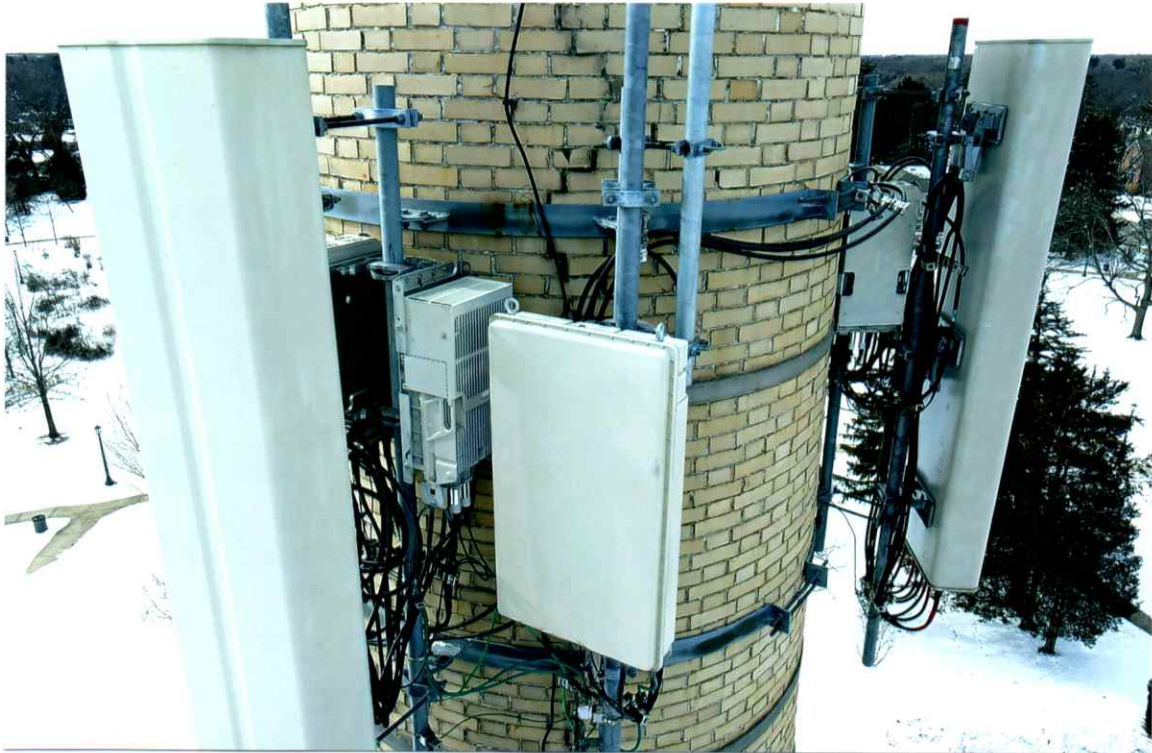
Photo 23. Overall good condition of the east side local to the upper level of antenna. All antennas and antenna support components were secure. Past repairs along the crack were sound.
