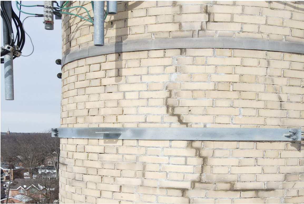
Photo 30. Close-up of the fair condition of the repaired crack (south side, 79' level).
