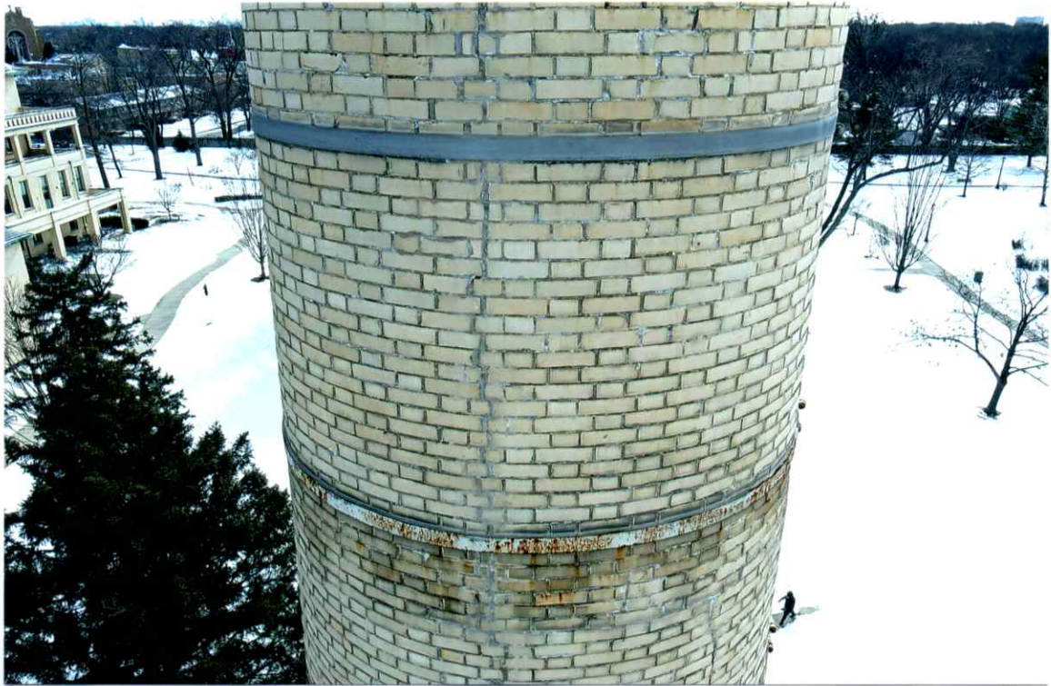
Photo 31. Fair exterior condition of the north side local to the 73' level. Mortar joints were weathered and recessed. Repairs to the crack were in fair condition (see Photo 39).
