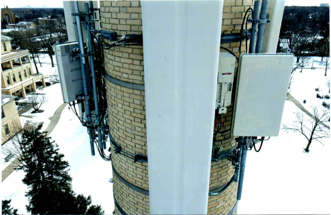
Photo 21. Overall good condition of the north side local to the lower level of antenna. All antennas and support components were secure. Mortar joints were only slightly weathered.
