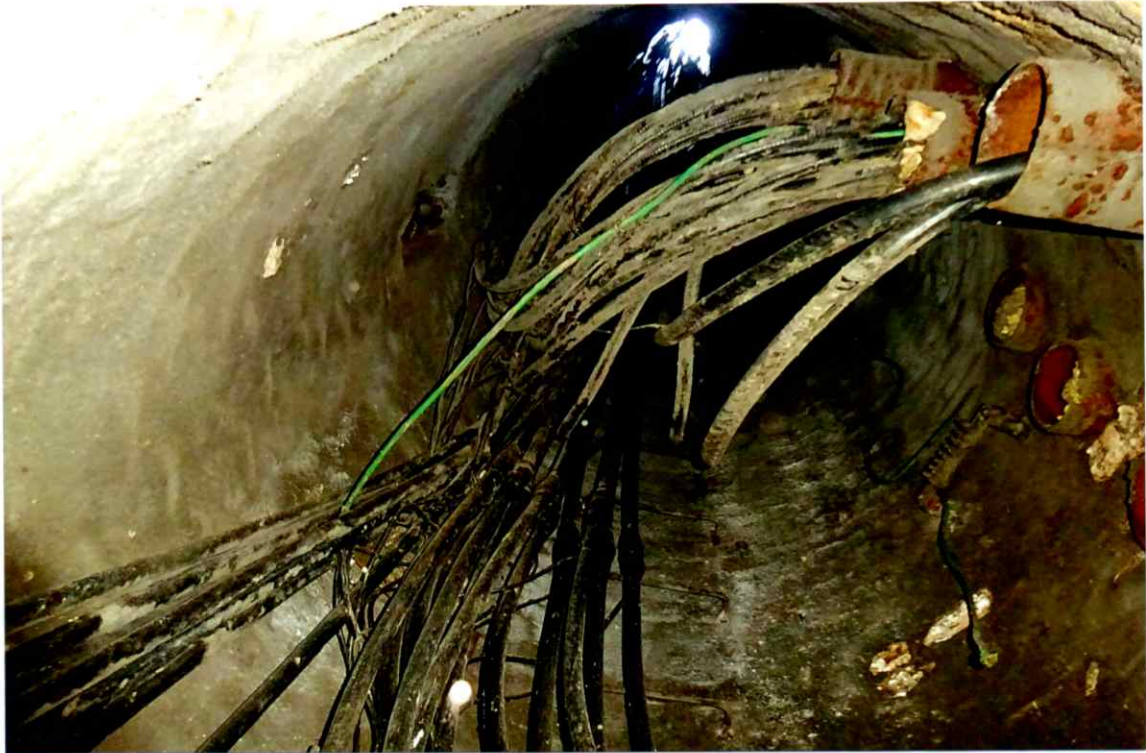
Photo 81. Good interior condition of the lower elevations looking up from the base. Note the numerous coaxial cables traversing up the chimney.
