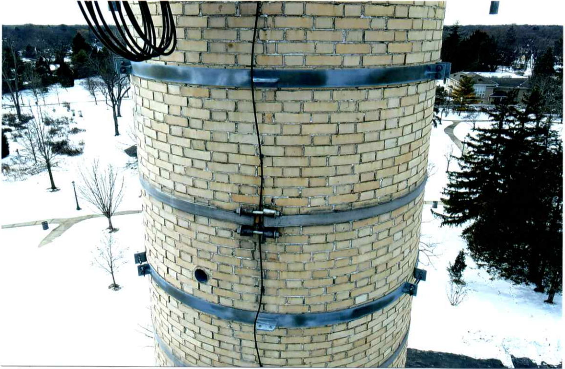
Photo 27. Fair exterior condition of the east side local to the 79' level. All bands were secure. Mortar joints were weathered and recessed.
