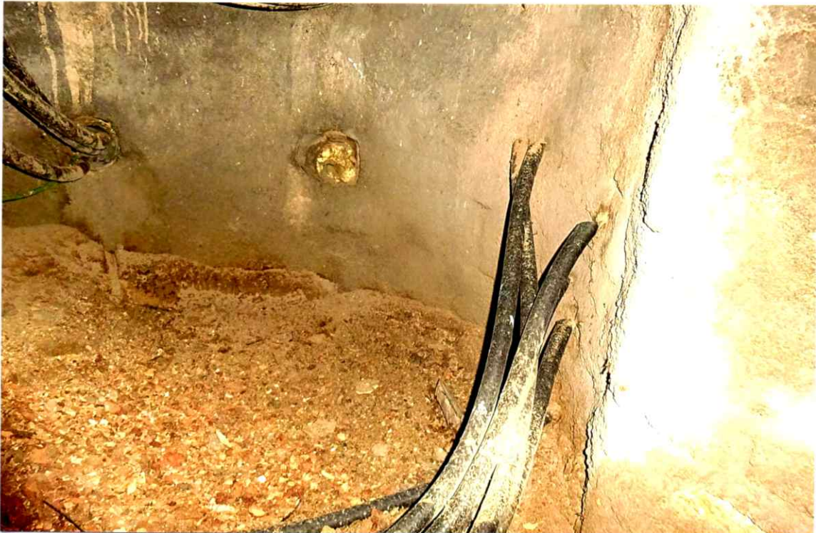
Photo 84. 8" of accumulated debris in the base (south side).
