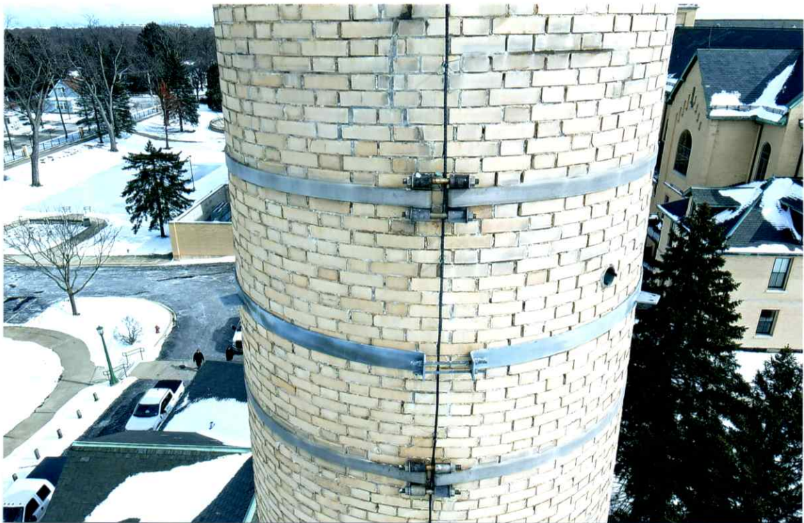
Photo 28. Fair exterior condition of the west side local to the 79' level. All bands were secure. Mortar joints were weathered and recessed.
