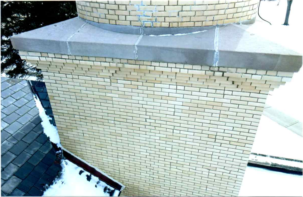
Photo 69. Good condition of the stone transition and corbelled square regions (29' level, north side). A few open and recessed mortar joints were observed.
