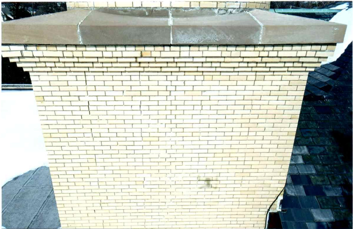
Photo 70. Good condition of the stone transition and corbelled square regions (29' level, south side). A few open and recessed mortar joints were observed.
