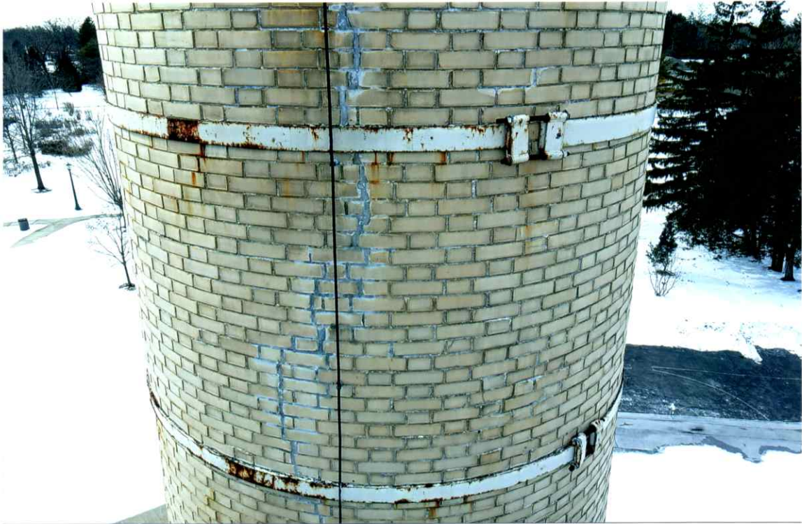
Photo 57. Good exterior condition of the east side local to the 44' level. Mortar joints were only slightly weathered. Repairs to the crack were sound (see Photo 60).
