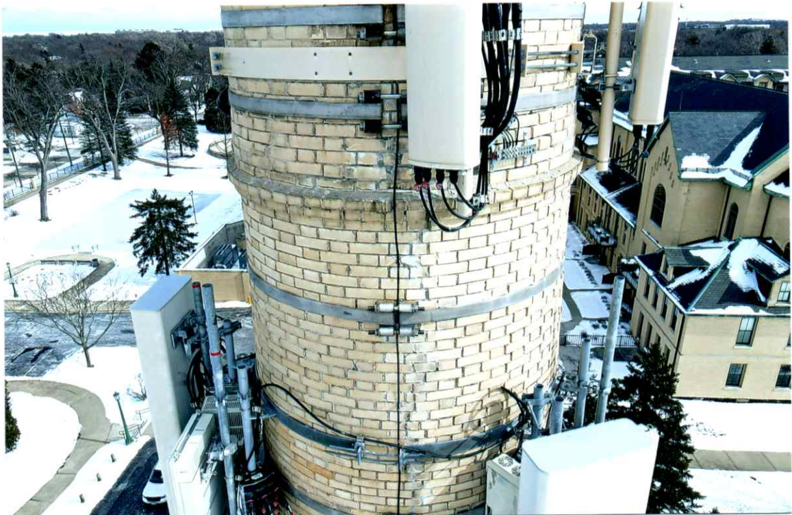
Photo 18. Fair exterior condition of mortar joints near the 93' level (west side). Past repairs to the crack were in fair condition in this region.
