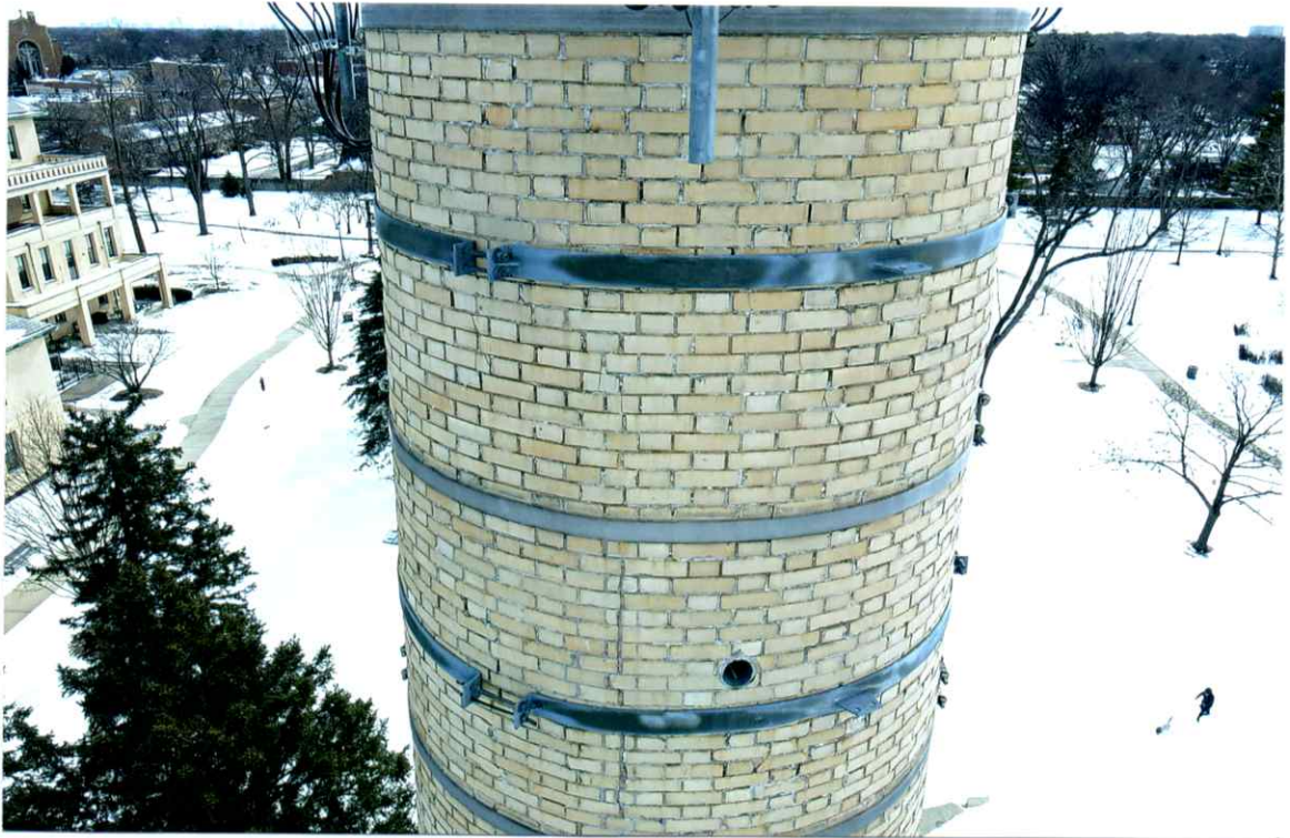
Photo 25. Fair exterior condition of the north side local to the 79' level. All bands were secure. Mortar joints were weathered and recessed.
