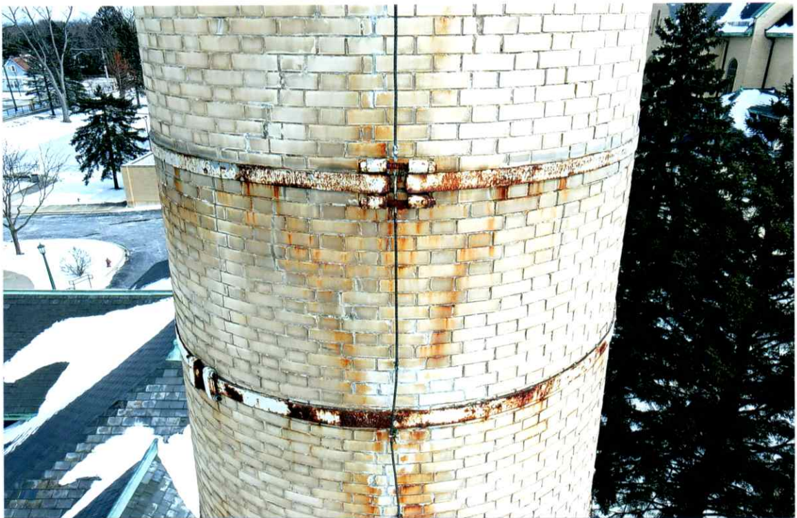
Photo 48. Good exterior condition of the west side local to the 56' level. Mortar joints were only slightly weathered. Repairs to the crack were sound.
