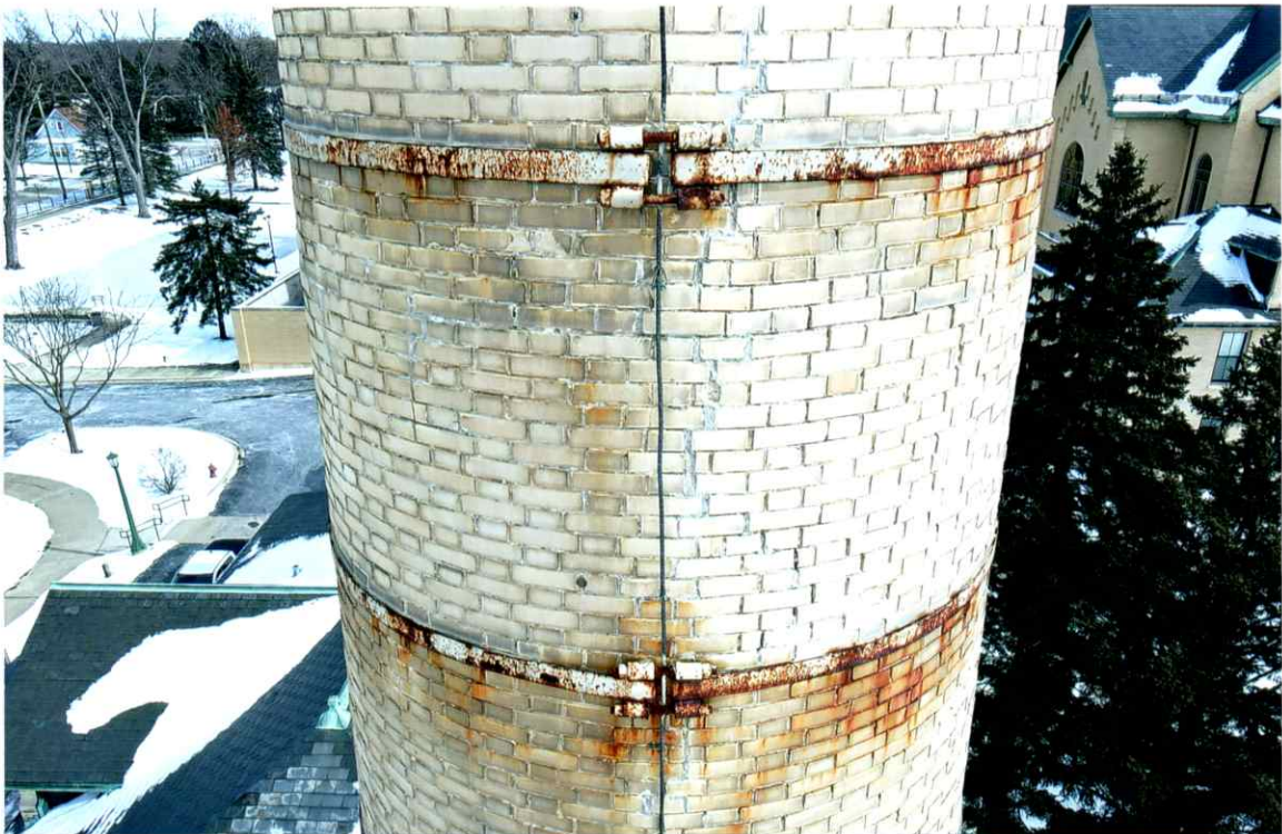
Photo 38. Fair exterior condition of the west side local to the 68' level. All bands were secure. Mortar joints were weathered and recessed.
