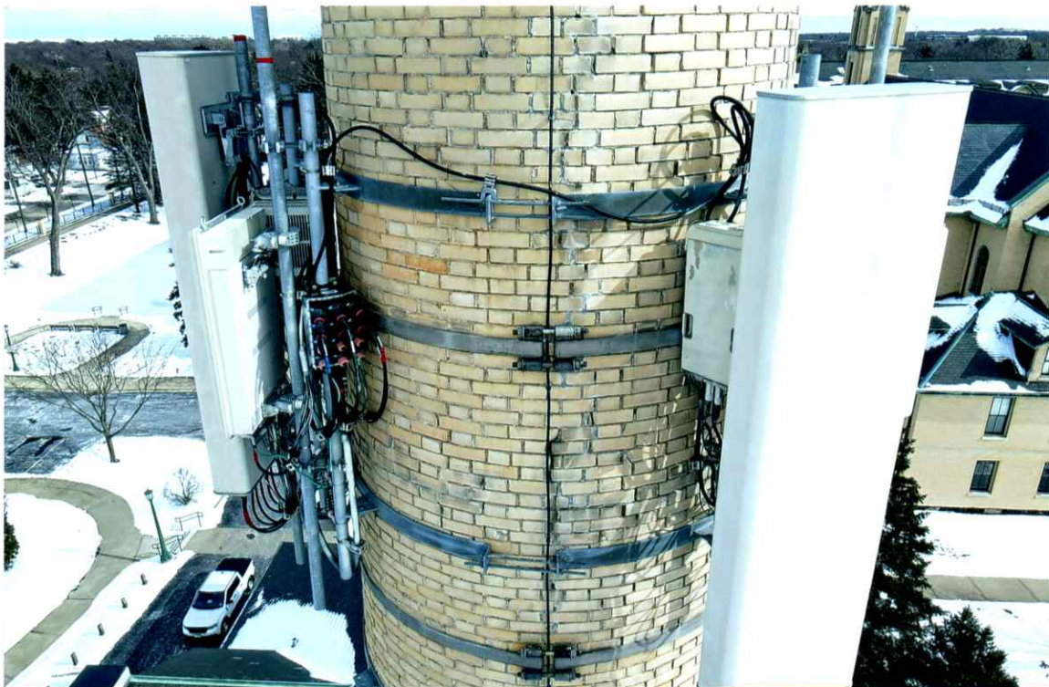
Photo 24. Overall good condition of the west side local to the upper level of antenna. Antennas and support components were secure. Past repairs along the crack were sound (Photo 29).
