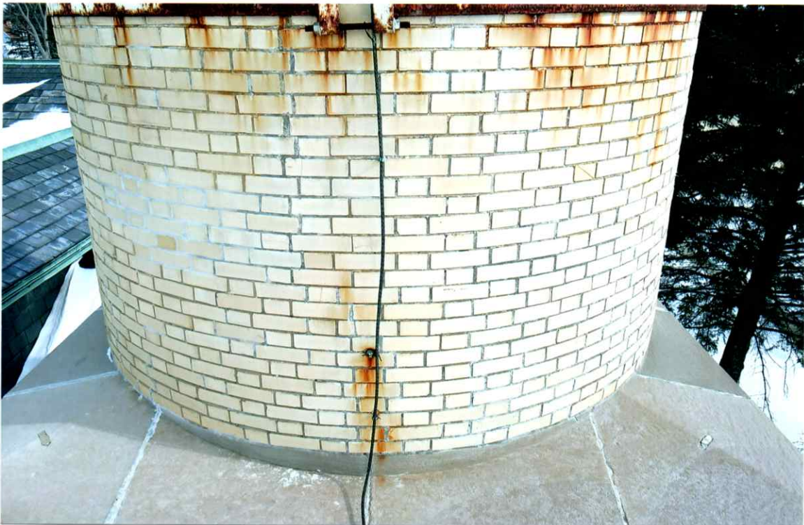
Photo 68. Good exterior condition of the west side local to the 32' level. Mortar joints were only slightly weathered.
