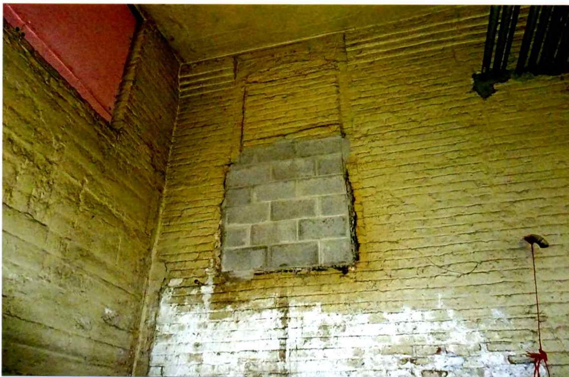
Photo 77. Good condition of the bricked and blocked up boiler duct opening (east side, sill near grade).
