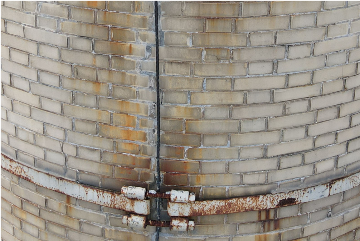
Photo 49. Close-up of the good condition of the repaired crack (east side, 61' level).
