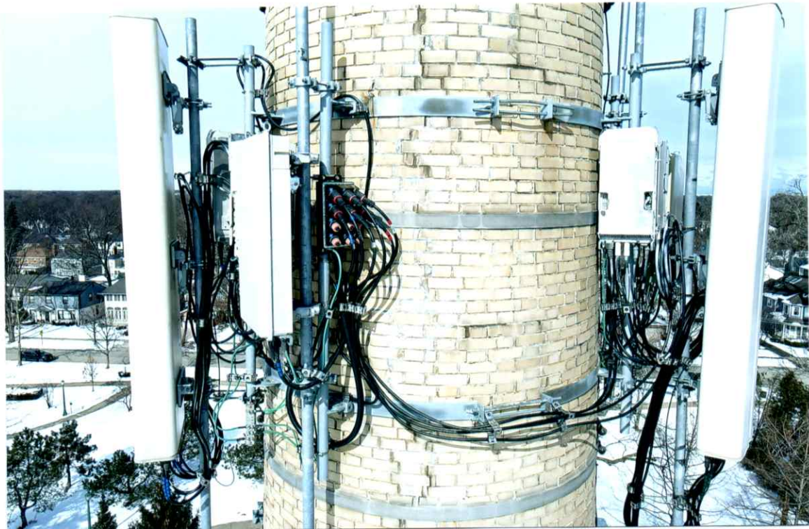
Photo 22. Overall good condition of the south side local to the lower level of antenna. All antennas and support components were secure. Past repairs along the crack were sound.
