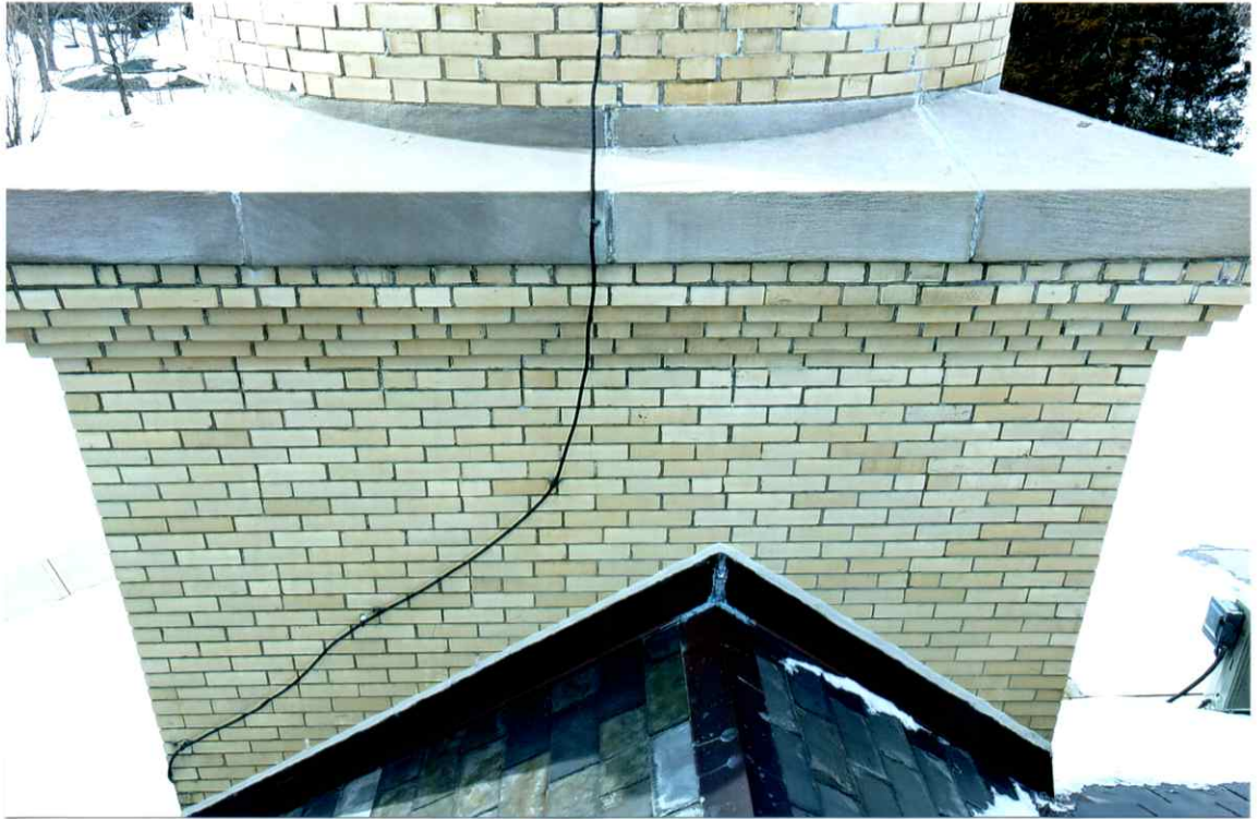
Photo 75. Good condition of the square region above the building roof (east side).
