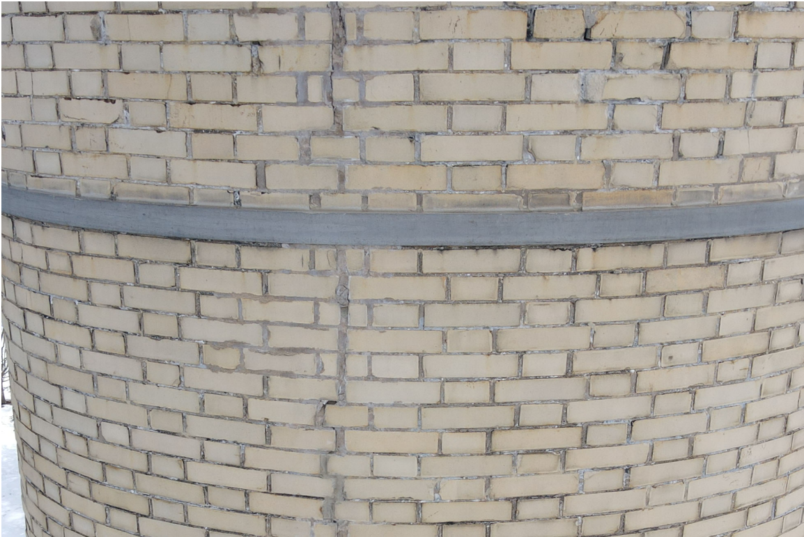
Photo 39. Close-up of the good condition of the repaired crack (north side, 73' level).
