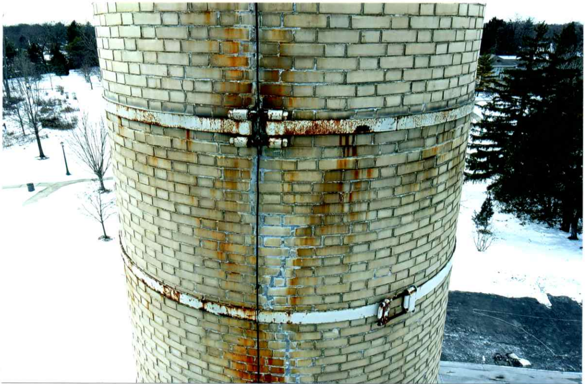
Photo 47. Good exterior condition of the east side local to the 56' level. Mortar joints were only slightly weathered. Repairs to the crack were sound.
