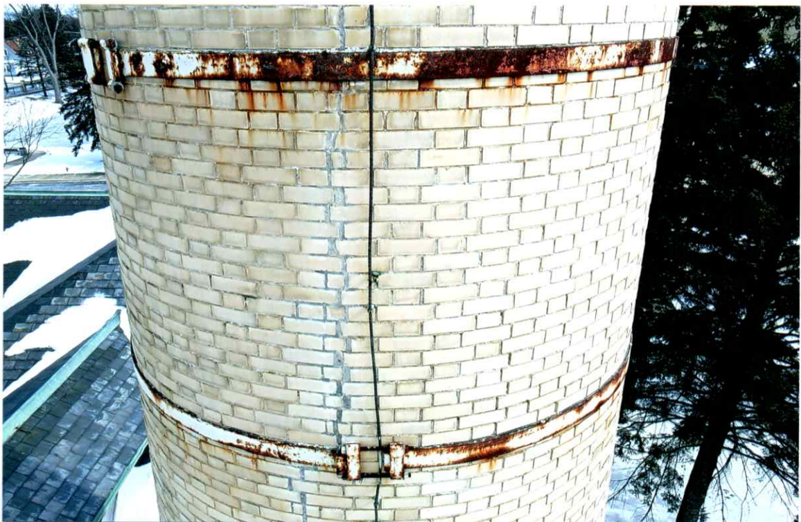
Photo 58. Good exterior condition of the west side local to the 44' level. Mortar joints were only slightly weathered. Repairs to the crack were sound.
