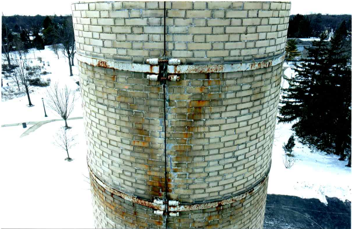
Photo 37. Fair exterior condition of the east side local to the 67' level. All bands were secure. Mortar joints were weathered and recessed.
