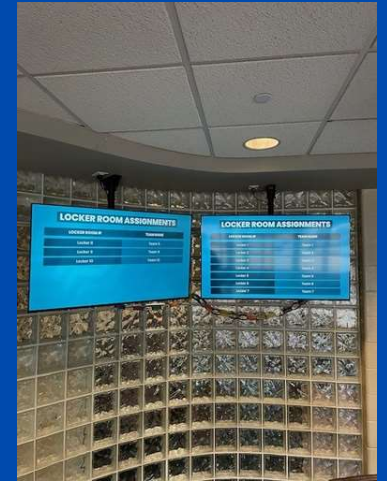
New Lobby Monitors
